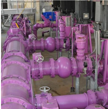
Fairfax County Water Reuse Facilities
