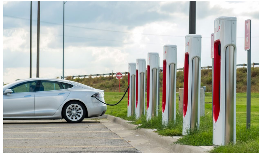
Electric Vehicle Charging
