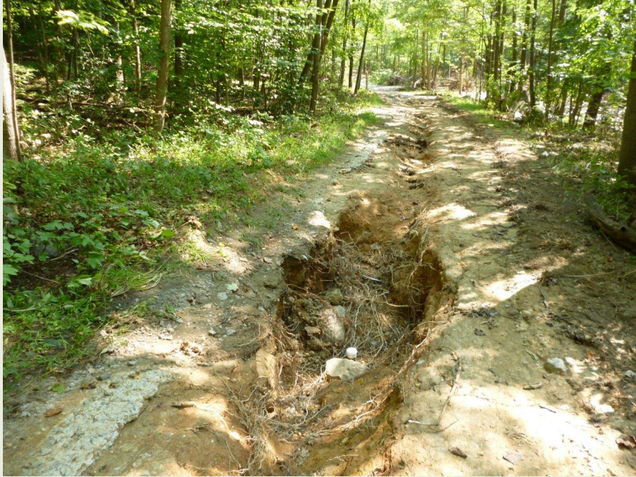
Heavily Damaged Gravel Section
