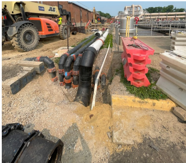
Figure 2-28: Temporary RSW line utilized to support Solids III Work
