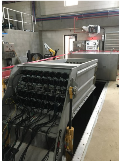
Figure 2-25: HH2 Building UV Disinfection System
