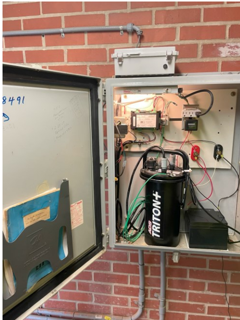
Figure 2-11: Pickett Road Flow Metering Station
