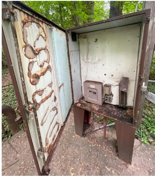
Figure 2-13: Ranger Road Flow Metering Station
