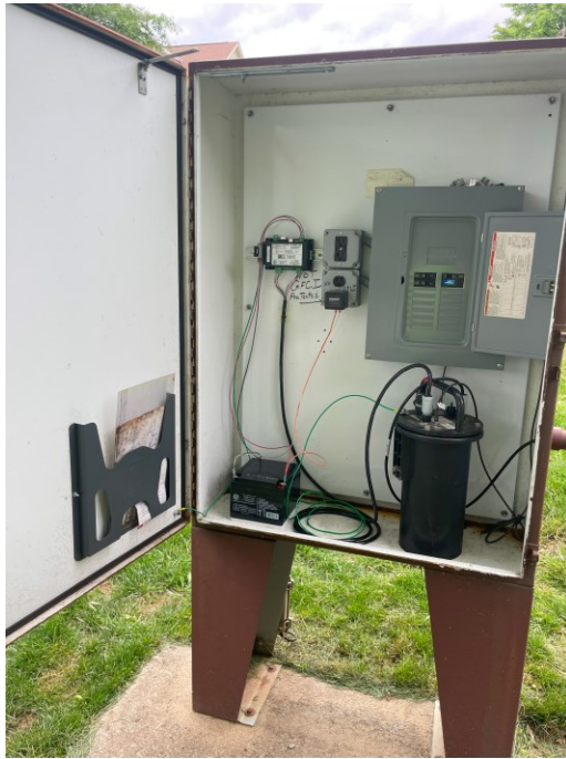
Figure 2-15: Rust Road Flow Metering Station
