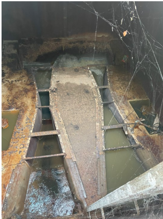
Figure 2-12: 12-inch Parshall Flume
