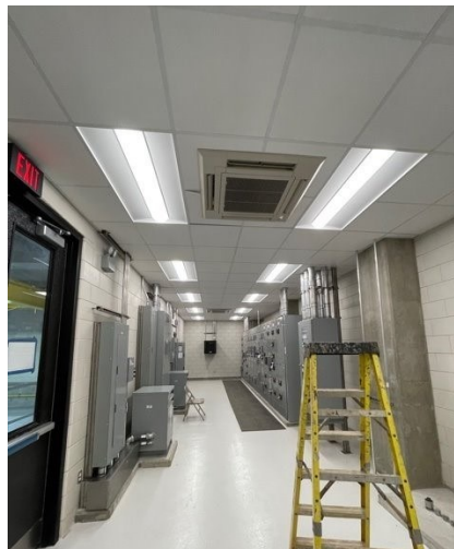
Figure 2-26: HH2 Building Electrical Room
