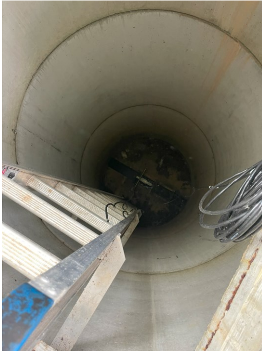
Figure 2-16: Rust Road 8-inch Palmer Bowlus
