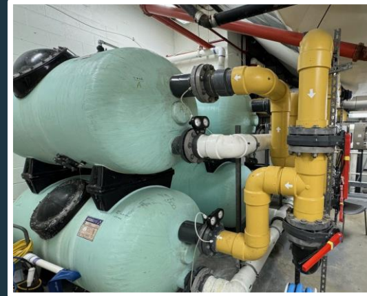
Existing Comp Pool Filters
