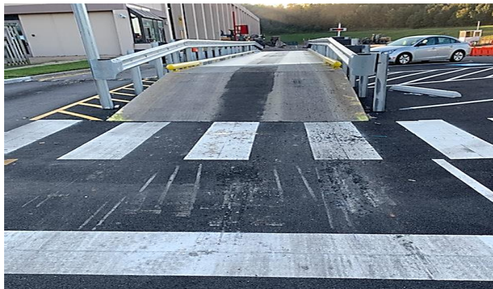
damage to scale approach
