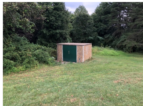
Figure 24: Irrigation Control Shed
