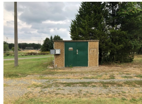
Figure 23: Electrical Control Shed
