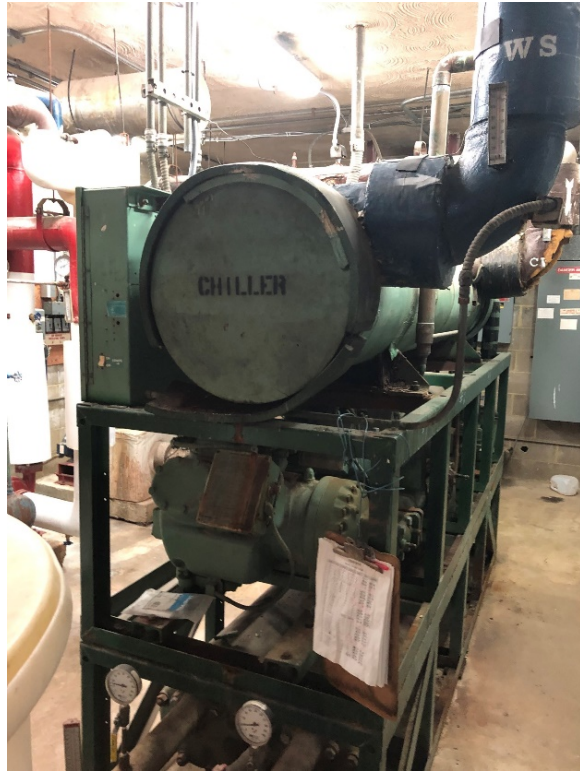
Audrey Moore Rec Center Chiller
