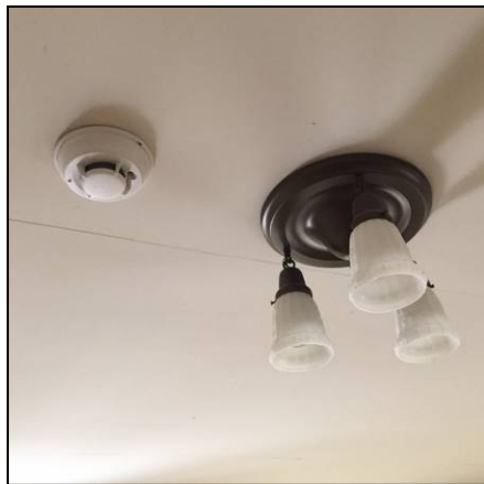
Image 22: Ceiling-Mounted Light Fixture
