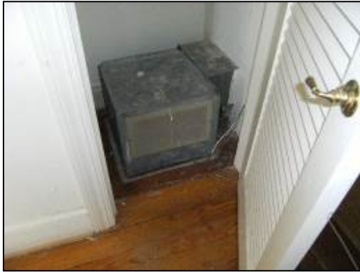
Image 8: Ductwork in Closet 112
