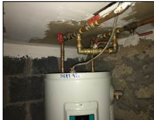
Image 5: Electric water heater
