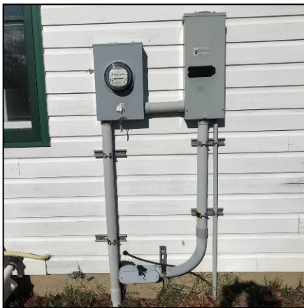
Image 18: Meter and Enclosed Circuit Breaker
