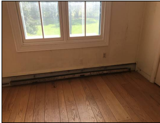
Image 6: Typical Damaged Radiator
