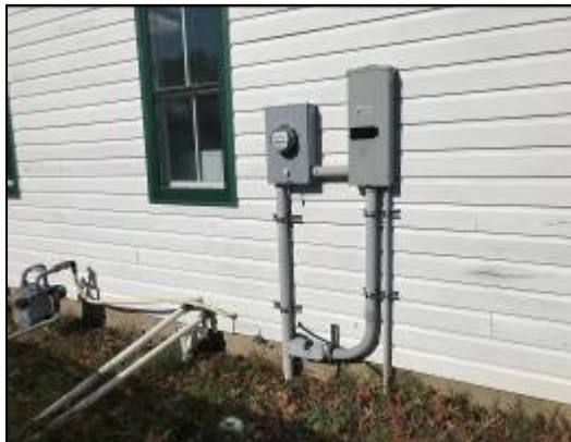
Image 4: Utilities meter outside
