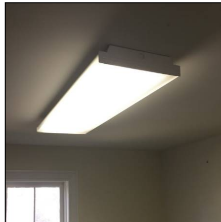
Image 23: Surface-Mounted Fluorescent Light Fixture
