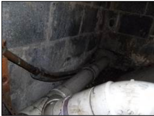
Image 10: Sanitary Sewer Piping
