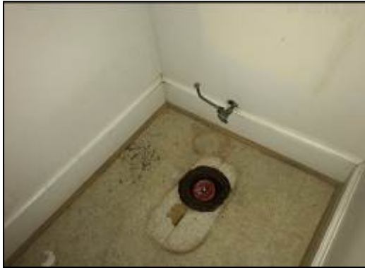
Image 14: Capped Sanitary Sewer Line
