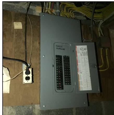
Image 19: Main Electrical Distribution Panelboard
