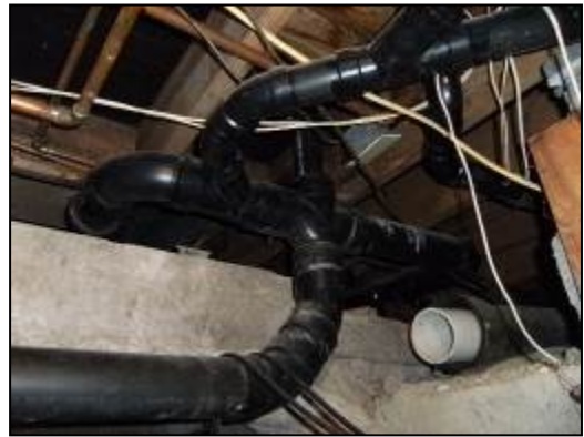
Image 11: Sanitary Sewer Piping
