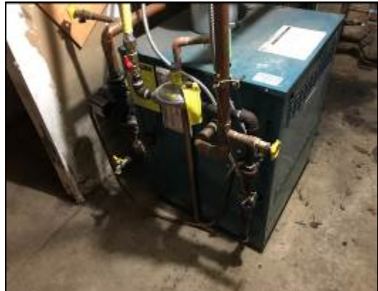
Image 3: Gas-fired Hydronic Boiler
