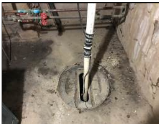
Image 12: Sump Pump Basement
