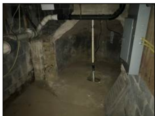
Image 13: Sump Pump Within Floor Drain
