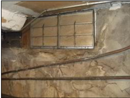
Image 2: Uninsulated Copper Piping
