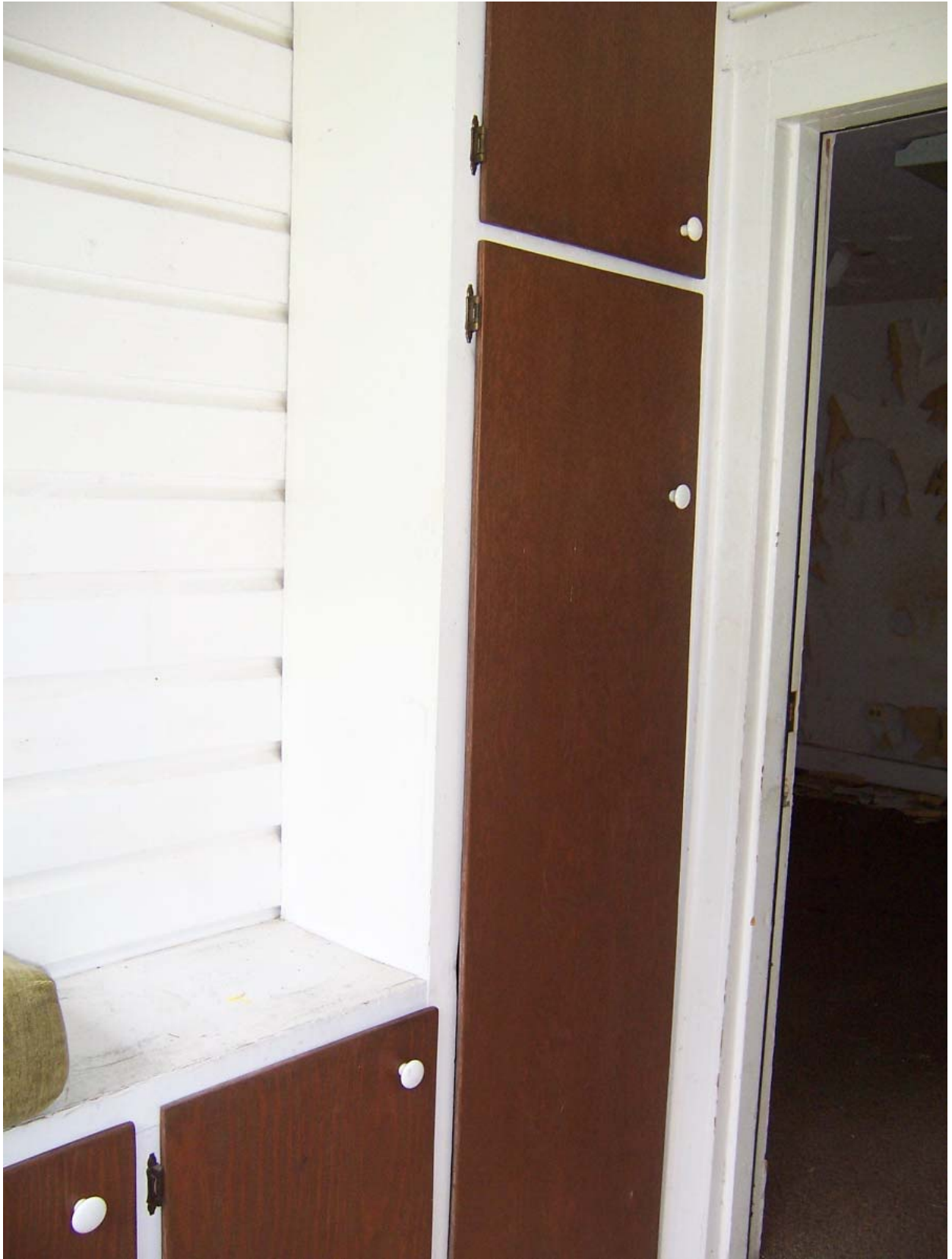
Existing Condition Photo B48: Stempson House First Floor Casework in Vestibule (Room 104)
