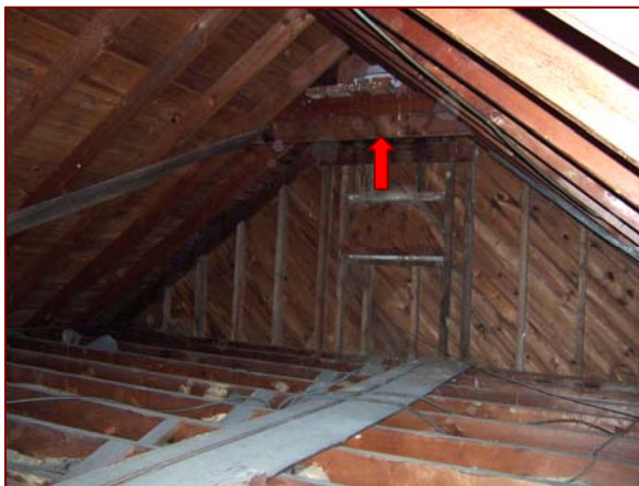
Image 3.21: Northern Chimney Extends into Attic and Rests on Platform, Red Arrow Points to Platform
