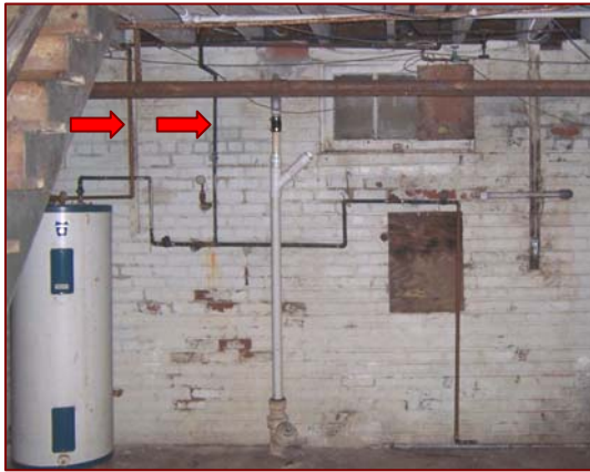
Image 3.88: Hot and Cold Water Pipes
