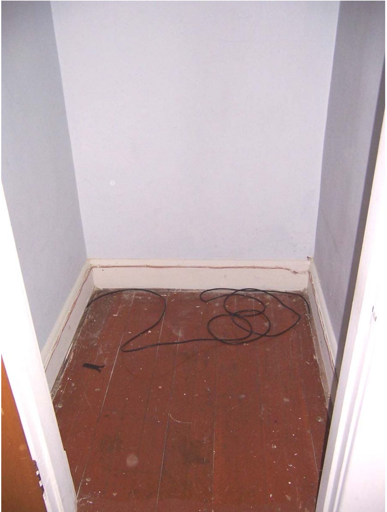
Existing Condition Photo B76: Stempson House Second Floor Closet for Room 202 (Room 208)
