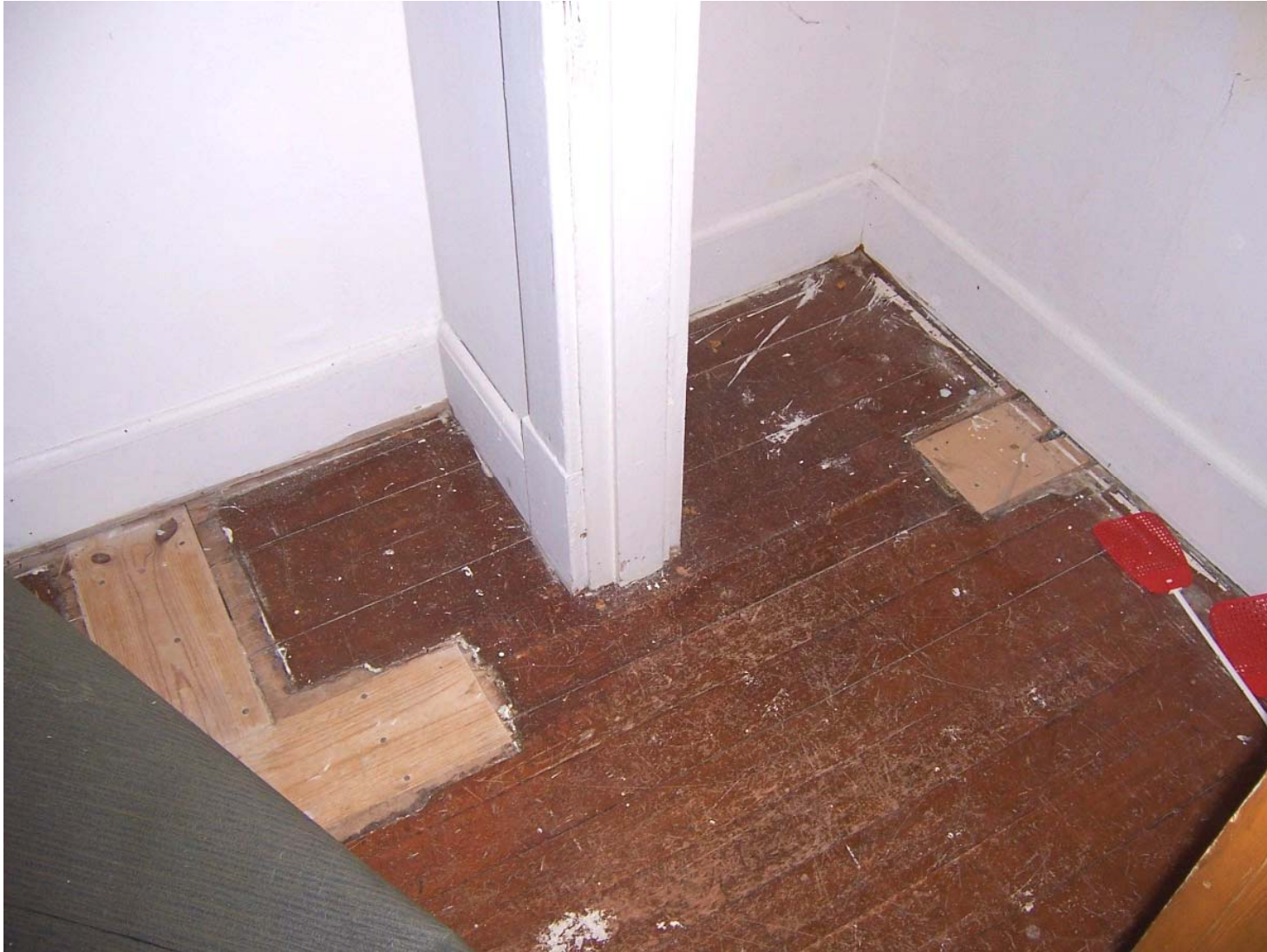
Existing Condition Photo B67: Stempson House Second Floor Nonextant Closet Location (Room 203)
