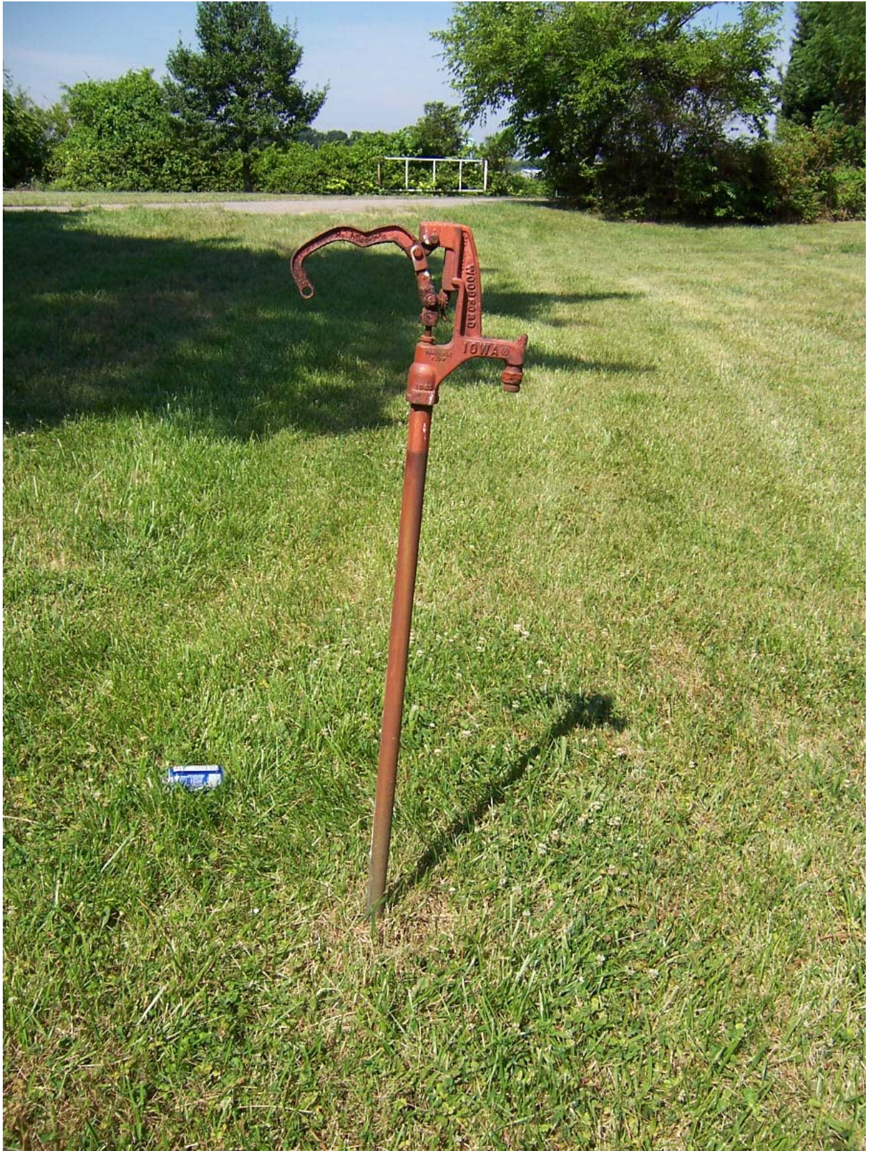
Existing Condition Photo B84: Stempson House Site Water Pump
