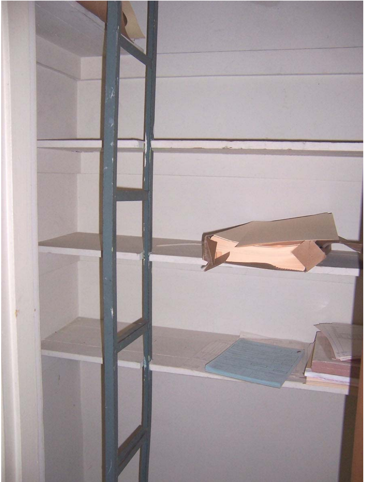
Existing Condition Photo B77: Stempson House Second Floor Closet Access to Attic (Room 209)
