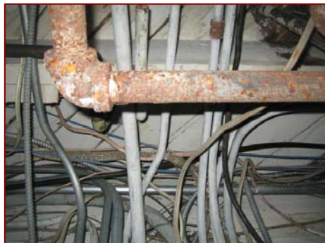
Image 3.14: Wiring Above Panel
