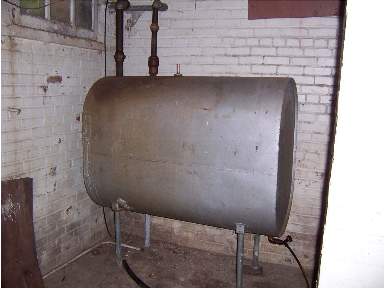
Existing Condition Photo B23: Stempson House Basement Fuel Tank
