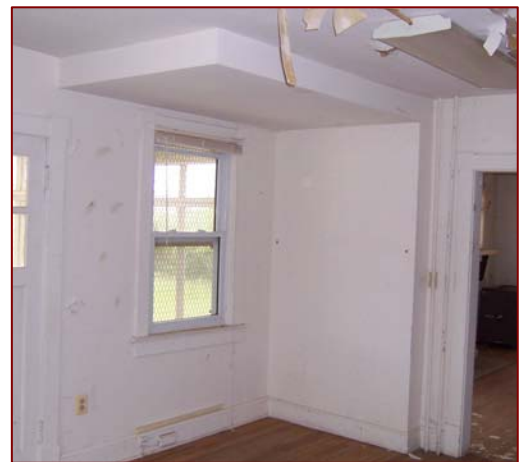
Image 3.62: Plumbing Bulkhead and Chase
