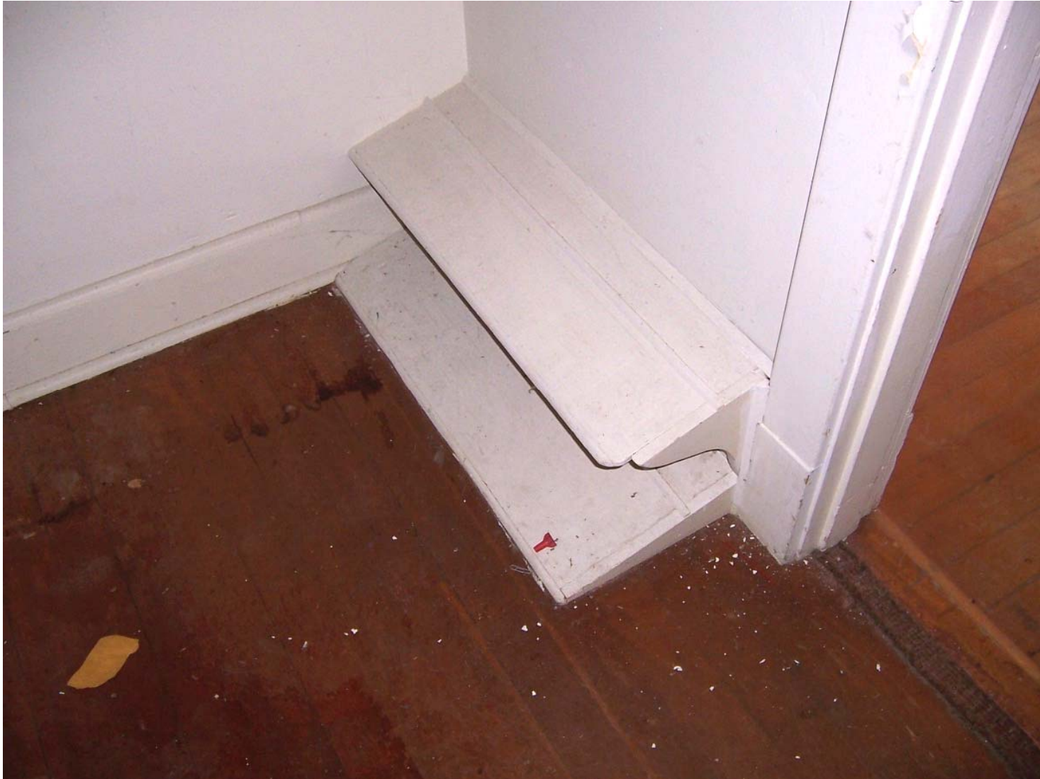
Existing Condition Photo B81: Stempson House Second Floor Closet for Room 200 (Room 211)
