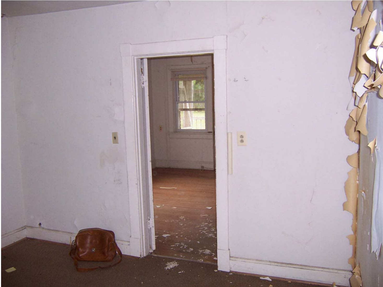
Existing Condition Photo B37: Stempson House First Floor Kitchen (Room 102) Doorway Into Room 103
