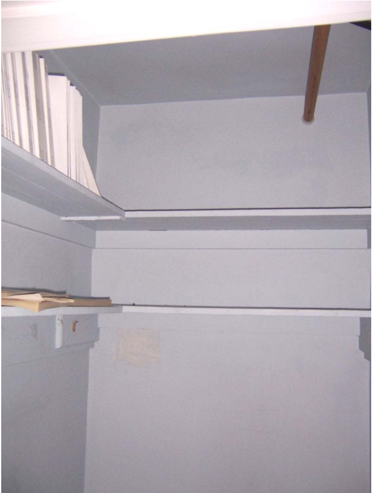
Existing Condition Photo B75: Stempson House Second Floor Closet for Room 202 (Room 208)
