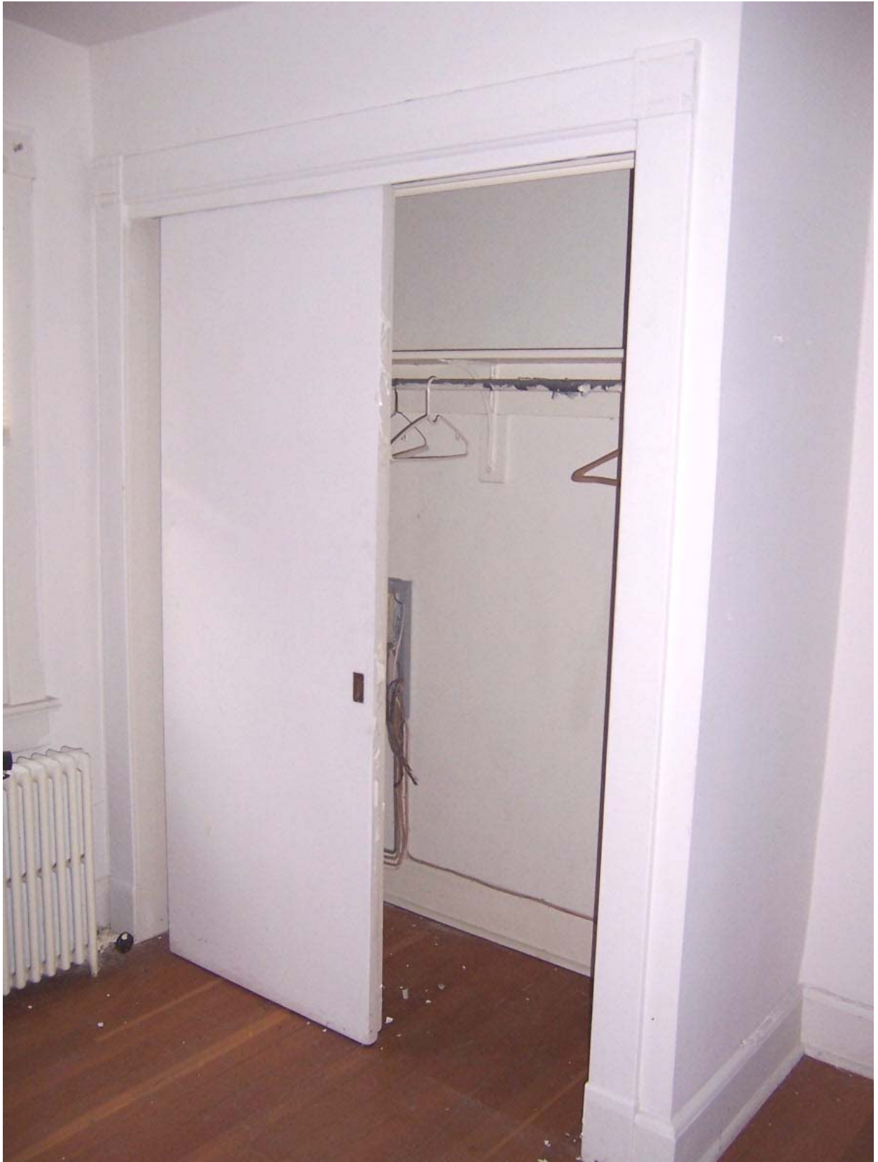
Existing Condition Photo B79: Stempson House Second Floor Closet for Room 201 (Room 210)
