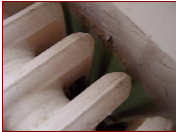
Image 3.49: Green Paint Behind Radiator
