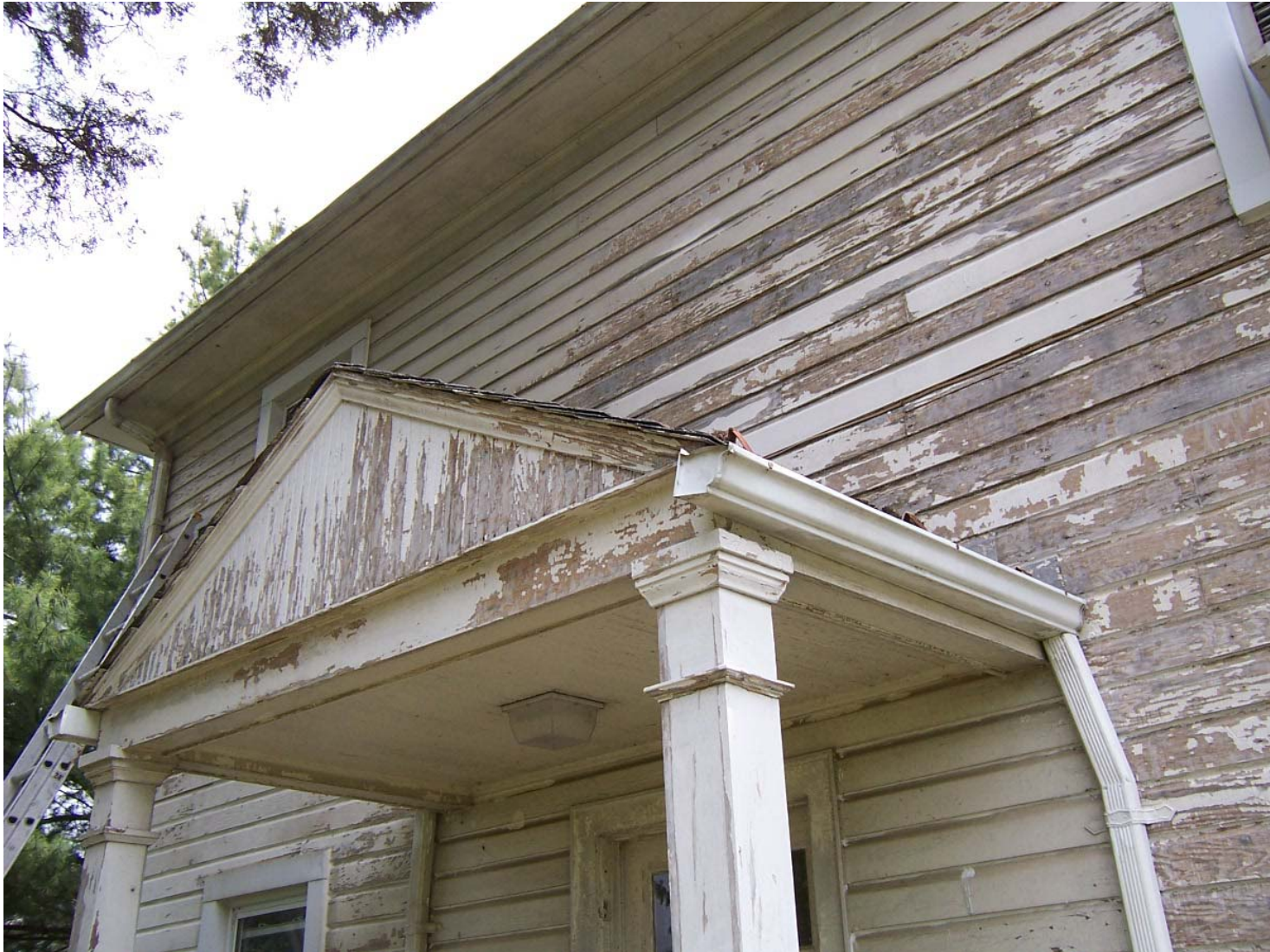
Existing Condition Photo B5: Stempson House Exterior West Porch Tympanium
