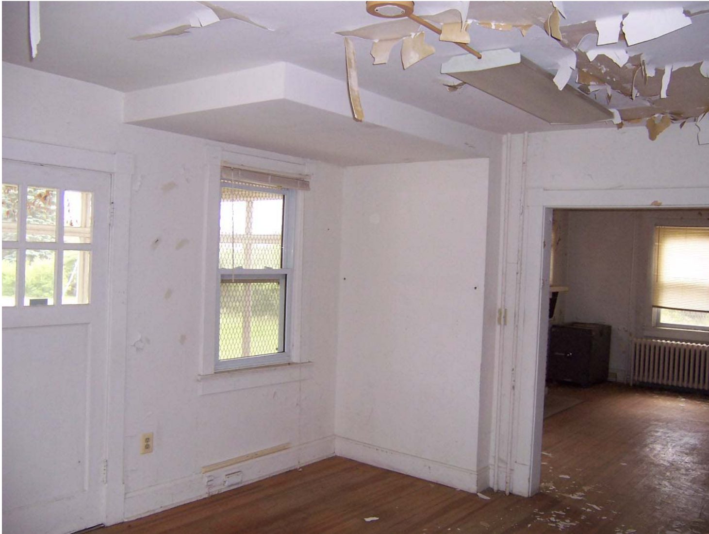
Existing Condition Photo B43: Stempson House First Floor Plumbing Bulkhead in Room 103
