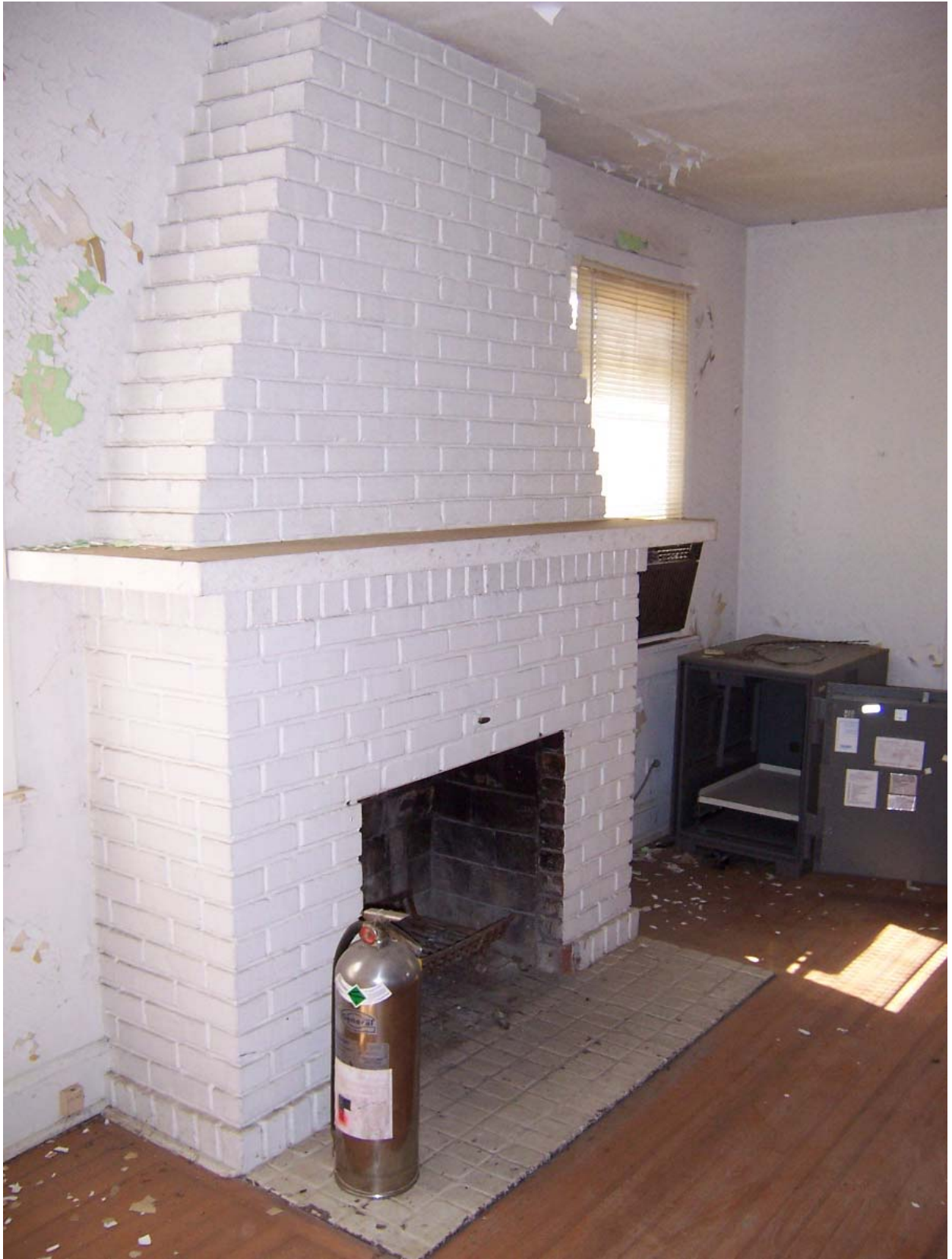
Existing Condition Photo B31: Stempson House First Floor Fireplace Brick Construction (Room 100)
