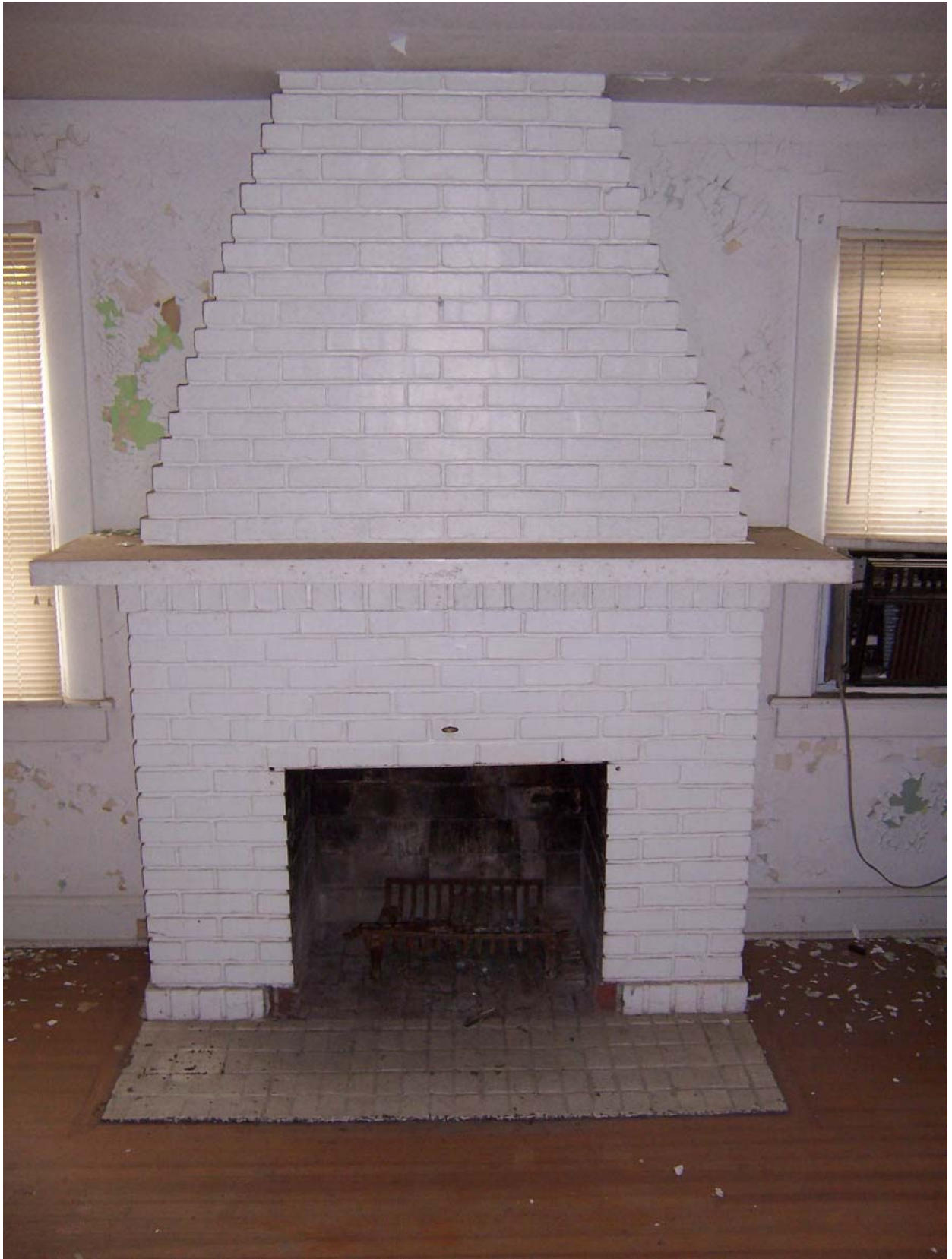
Existing Condition Photo B30: Stempson House First Floor Fireplace in Living Room (Room 100)
