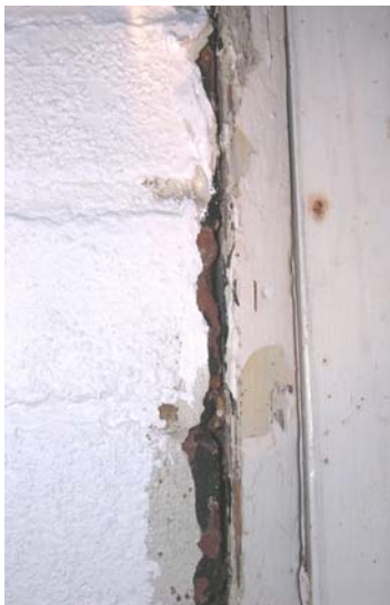
Image 3.98: Broken Brick at Door Penetration (D01)
