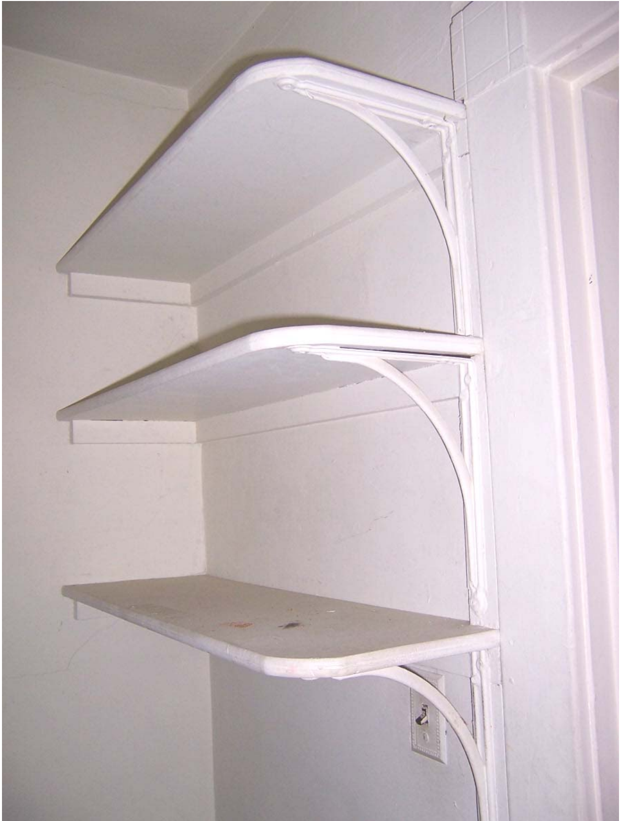
Existing Condition Photo B80: Stempson House Second Floor Closet for Room 200 (Room 211)
