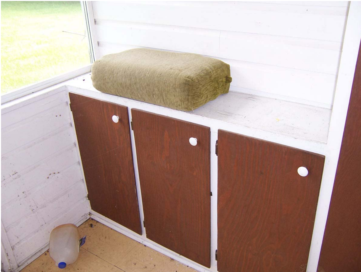
Existing Condition Photo B47: Stempson House First Floor Casework in Vestibule (Room 104)
