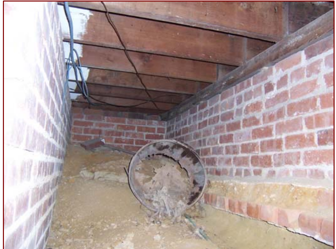
Image 3.7: Joist Bearing Foundation Wall Belled Out at Base
