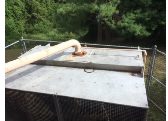
HVAC systems nearing end of service life
