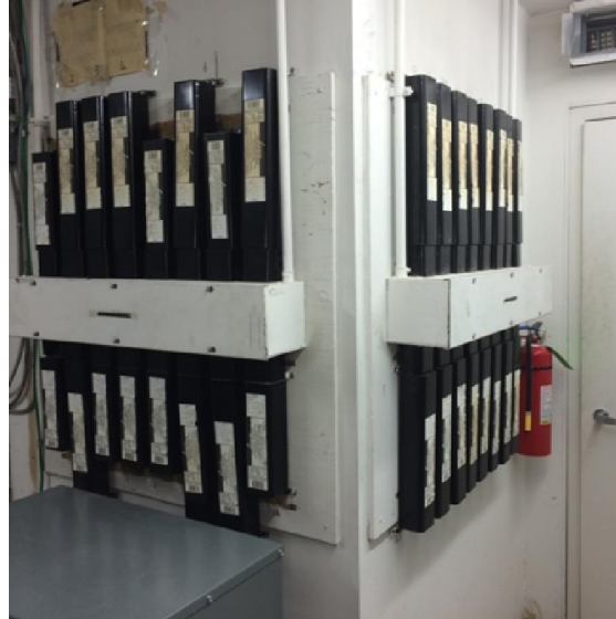
Old light ballast system, outdated, not energy efficient
