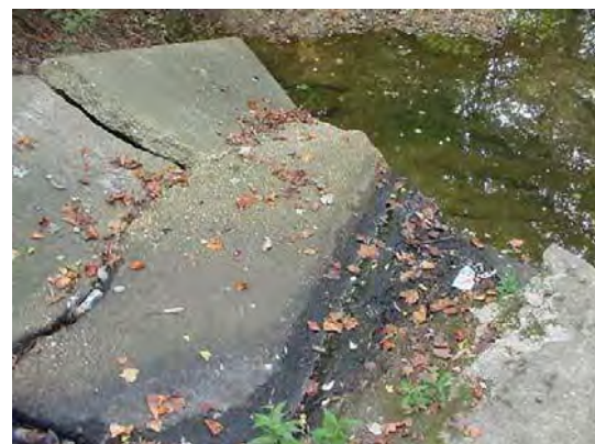
Broken concrete at the end of the channel
