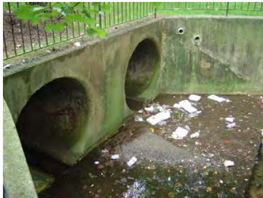
Outlets filled with trash and debris
