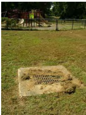
Detention berms can encircle grate inlets like this one to slow flows
