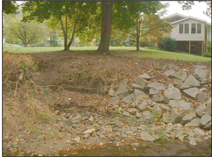
Bank erosion and inadequate buffer along Indian Run
