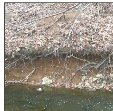
Streambank erosion at Lower Holmes Run
