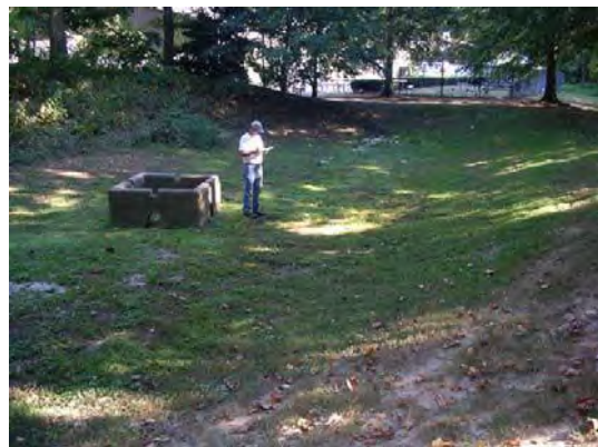
SWM pond and control structure
