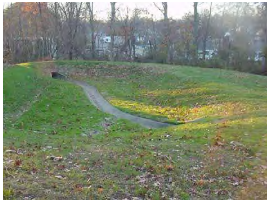
SWM dry pond
