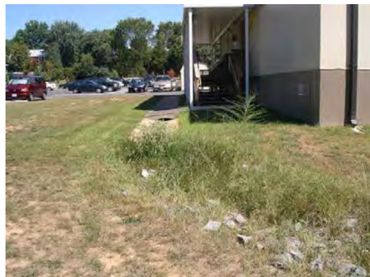
Convert concrete ditch to linear bioretention area and collect water from downspouts
