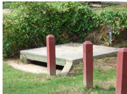
Stormwater inlet in park
