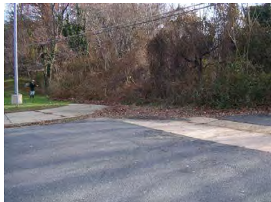
Stormwater pipe draining area south of Yellowstone Dr outlets in woods adjacent to school parking lot
