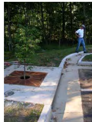
Newly constructed parking lot with existing tree box filter, underdrain, and infiltration
