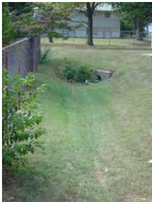
Grassy swale leading to inlet
