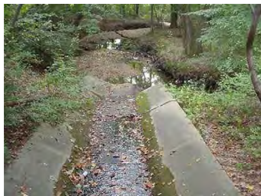
Existing concrete ditch at stormwater outfall
