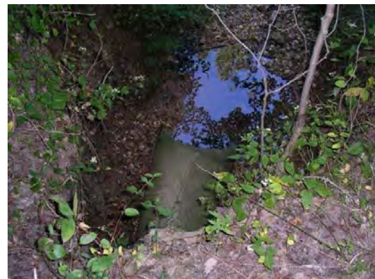
View of eroded outfall from above
