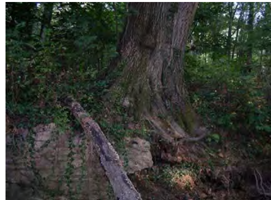
Evidence of bank erosion
