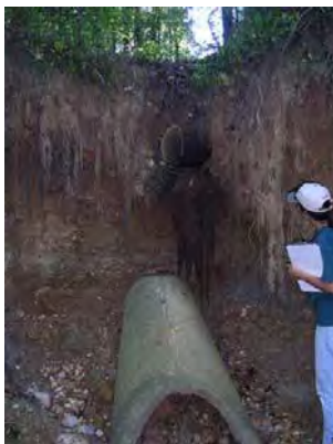
Divert stormwater into off-line bioretention areas above this eroded pipe outfall
