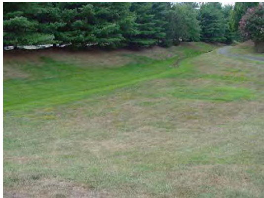
SWM dry pond
