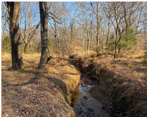
Widening channel with actively eroding banks and lack of trees.
