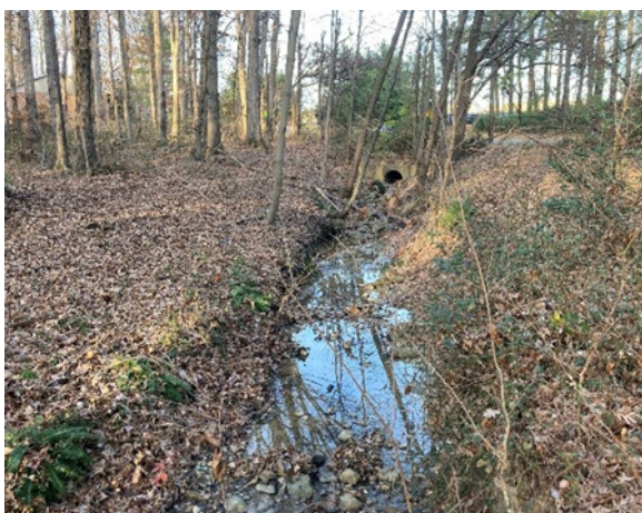
Incised and widening outfall channel.
