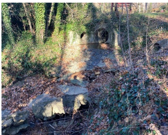
Three outfalls at upstream end of reach with failing apron structure.
