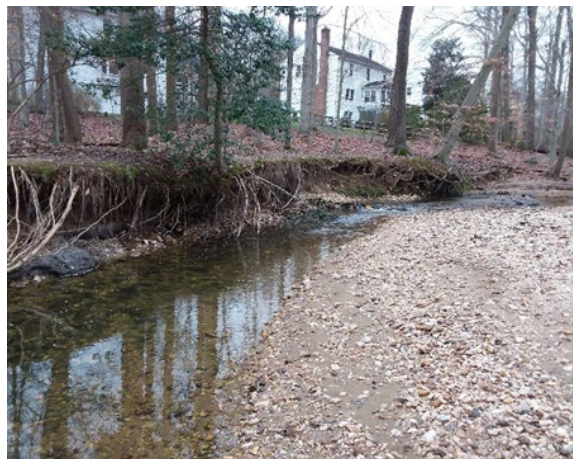
Widened stream channel with active bank erosion and an alignment nearing private properties.
