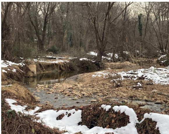
Entrenched, widening stream channel impeding on infrastructure; large supply of streambed material.
