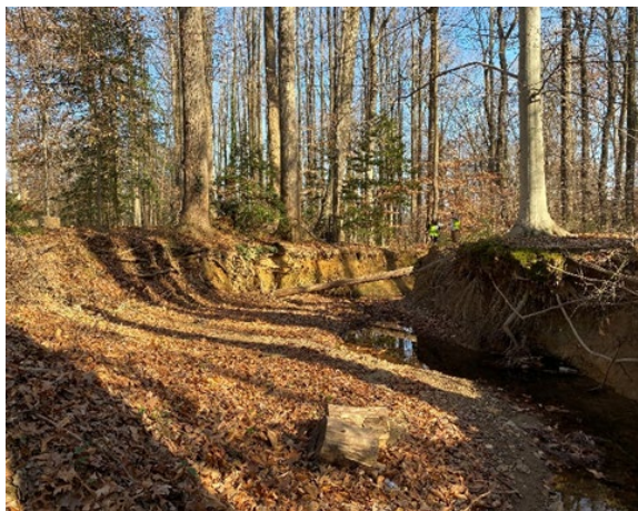
Widening channel with actively eroding banks.
