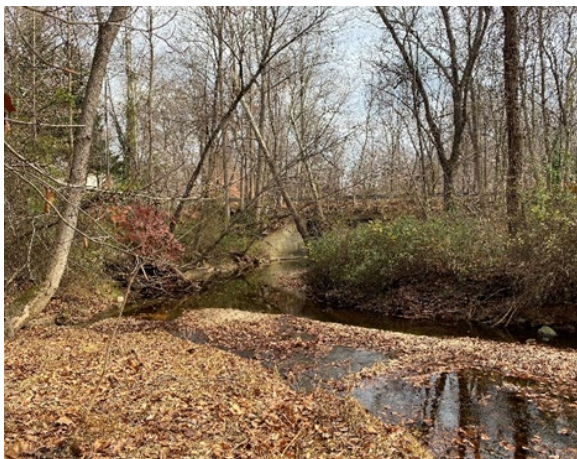
Widening stream channel with poor alignment into downstream culvert; large supply of sediment and streambed material in front of
