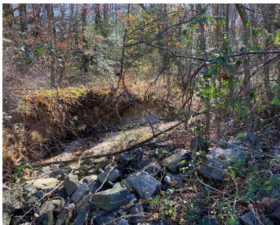
Degraded outfall channel.
