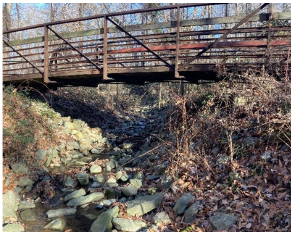
Large pedestrian foot bridge spanning stream where elevation and plan form are a constraint.
