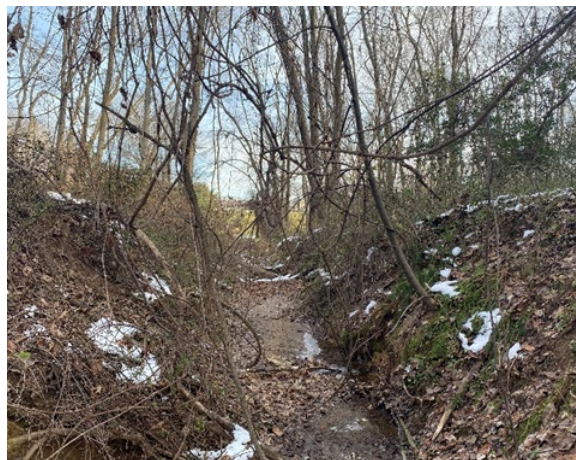
Incised, widening outfall channel.
