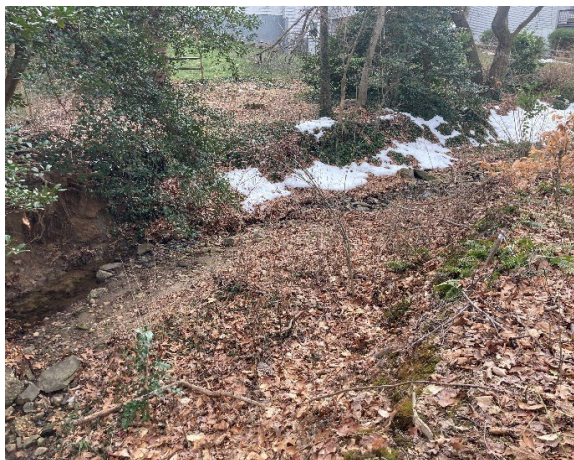
Channel alignment impeding on existing sewer infrastructure.
