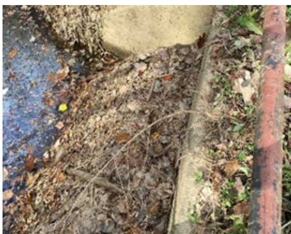
Clogged low-flow orifice.
