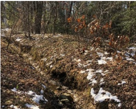
Degraded outfall channel.
