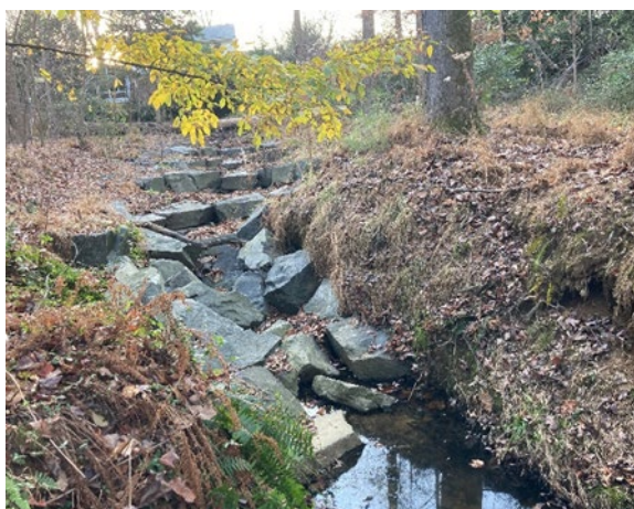
Previously stabilized outfall channel with grade control failure.
