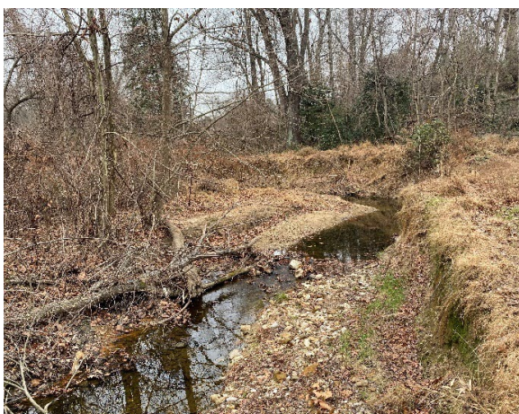
Incised and widening channel beginning to encroach on the sewer.
