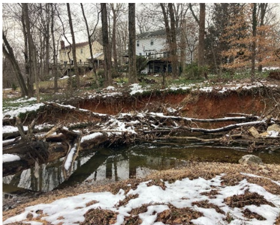
Stream channel impeding on private property.
