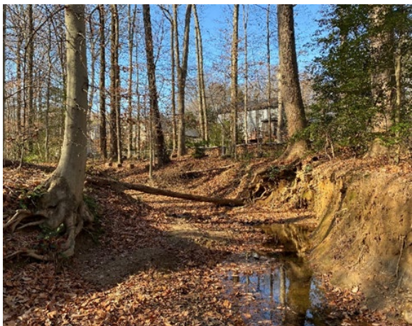
Widening channel with actively eroding banks near private properties.
