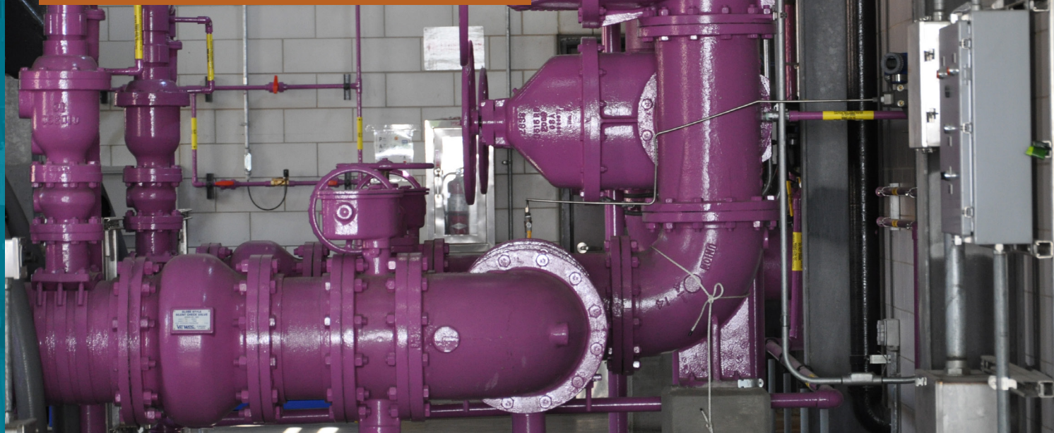
Water reuse pipes at Noman M. Cole, Jr. Pollution Control Plant.
