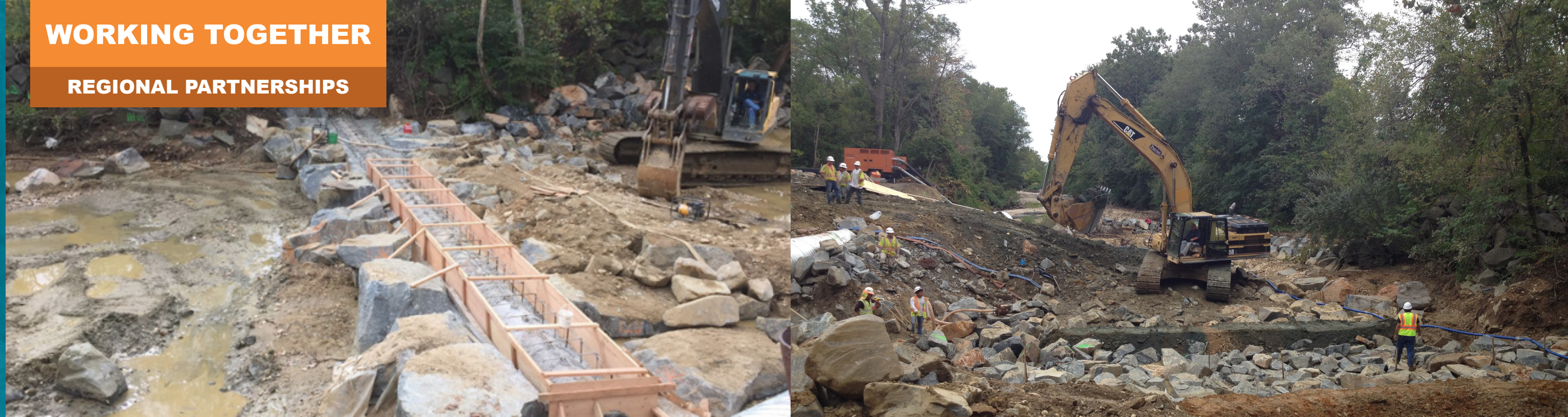
South Van Dorn Sanitary Sewer Stream Crossing.
