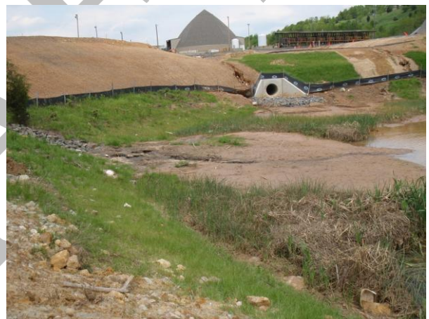
Figure 2-41: Erosion and heavy sedimentation in several ponds southeast of the intersection of I-66 and Fairfax County Parkway
