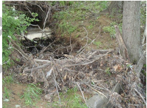
Figure 2-13: Debris obstruction and headcut near Clifton Rd. and Cedar Ridge Dr.
