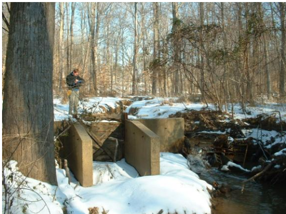
Figure 2-29: Moderate to Severe Obstruction on Little Rocky Run
