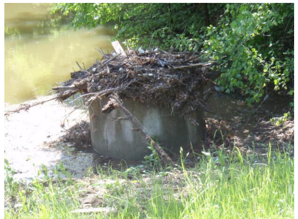
Figure 2-26: Pond riser structure is covered with debris near Compton Heights Circle
