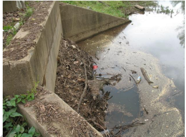
Figure 2-40: Obstruction in pond near Tractor Lane
