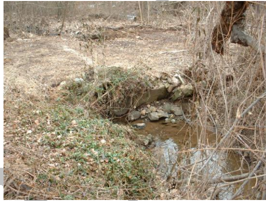
Figure 2-19: Pipe Impact upstream of Union Mill Road
