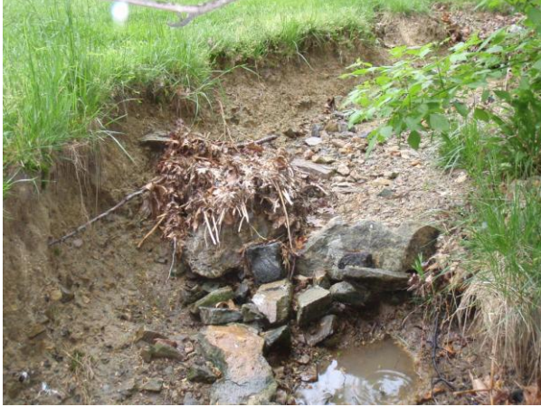
Figure 2-20: Severe erosion occurring at the end of a concrete trickle ditch in the Little Rocky Run subdivision (Battle Rock Drive)
