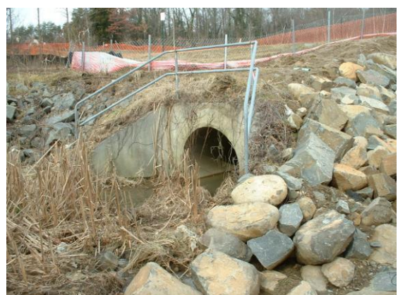
Figure 2-32: Crossing Impact on Tributary upstream of Lee Highway
