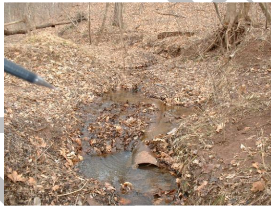
Figure 2-7: Pipe Impact near confluence with Bull Run
