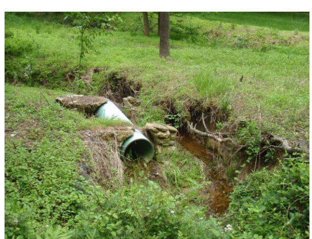
Figure 2-15: Pipe Impact near Clifton Rd. and Cedar Ridge Dr.
