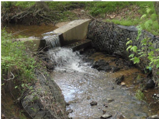
Figure 2-14: Manmade obstruction near Clifton Rd. and Cedar Ridge Dr.
