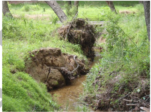
Figure 2-9: Bank erosion in excess of 3ft on small tributary near Cedar Ridge Drive
