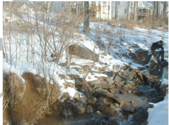
Figure 2-30: Moderate to Severe Pipe Impact on Little Rocky Run
