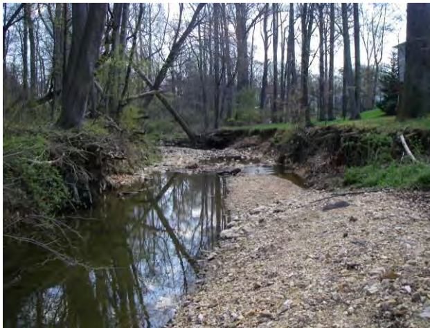
Site Photo: Over-widened channel with severe bank erosion
