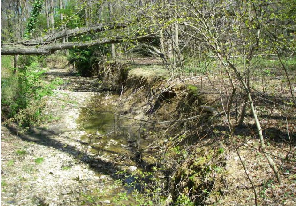
Site Photo: Over-widened channel with moderate to severe erosion
