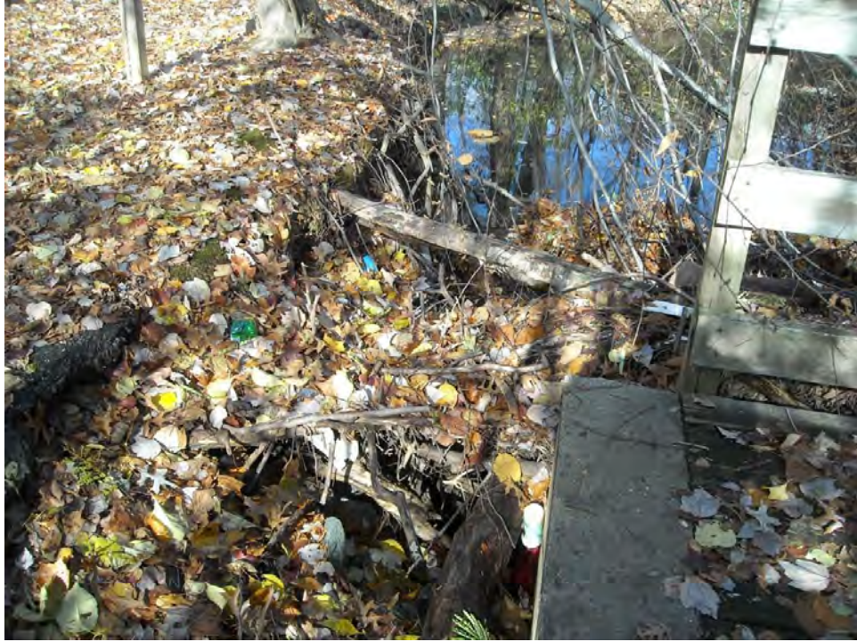
Figure 1: Eroded banks and scour at a footbridge near Lee Highway
