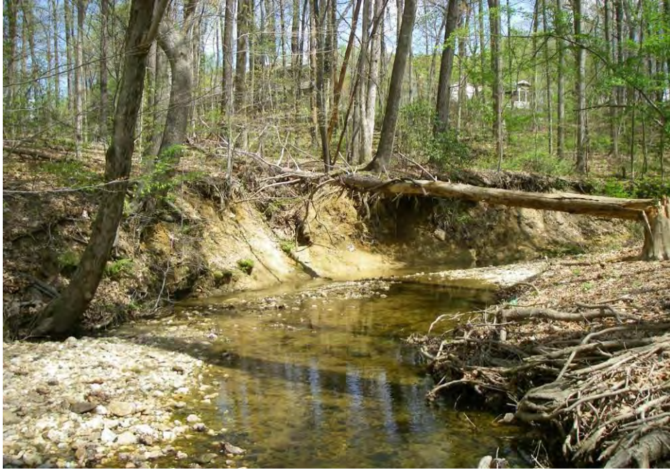
Site Photo: Moderate to severe erosion on outside meander bends
