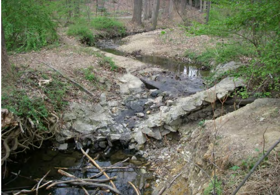
Site Photo: Exposed sanitary sewer casing and headcut
