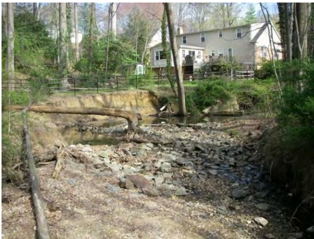
Site Photo: Eroded downstream channel starts at culvert near Guinevere Drive and Launcelot Way
