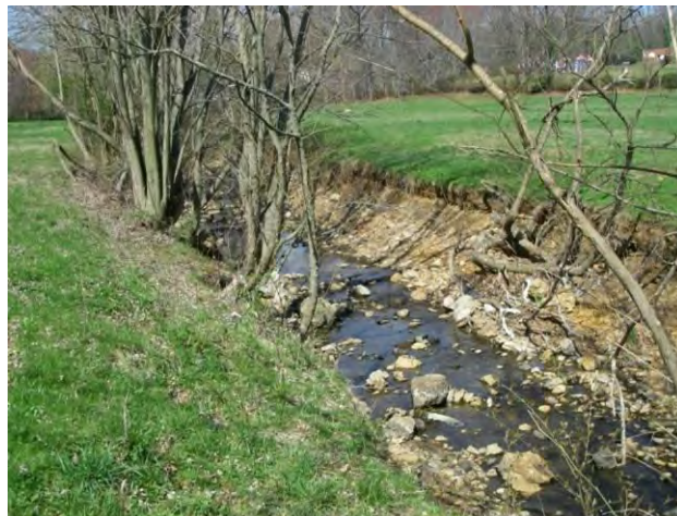
Site Photo: Upstream end with moderate erosion and no riparian buffer
