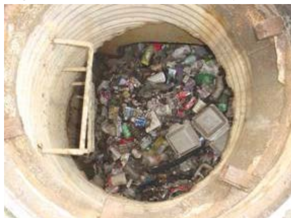
Figure 4-28: Catch basin (Source: Fairfax County)
