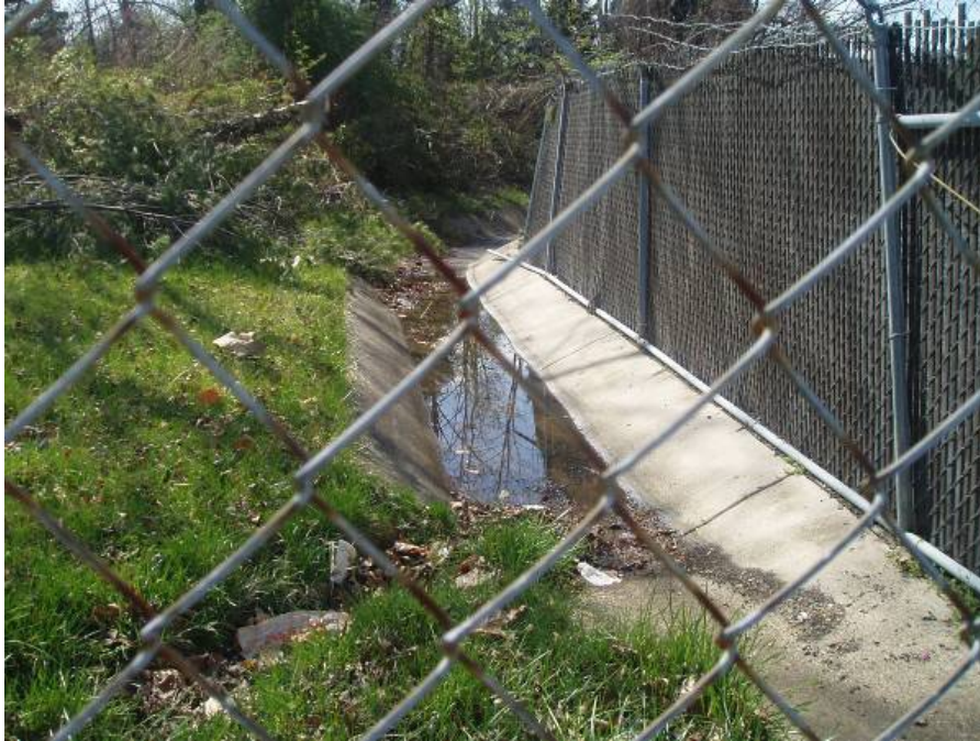
Site photo: AC9550B, concrete channel to be replaced with a vegetated swale.
