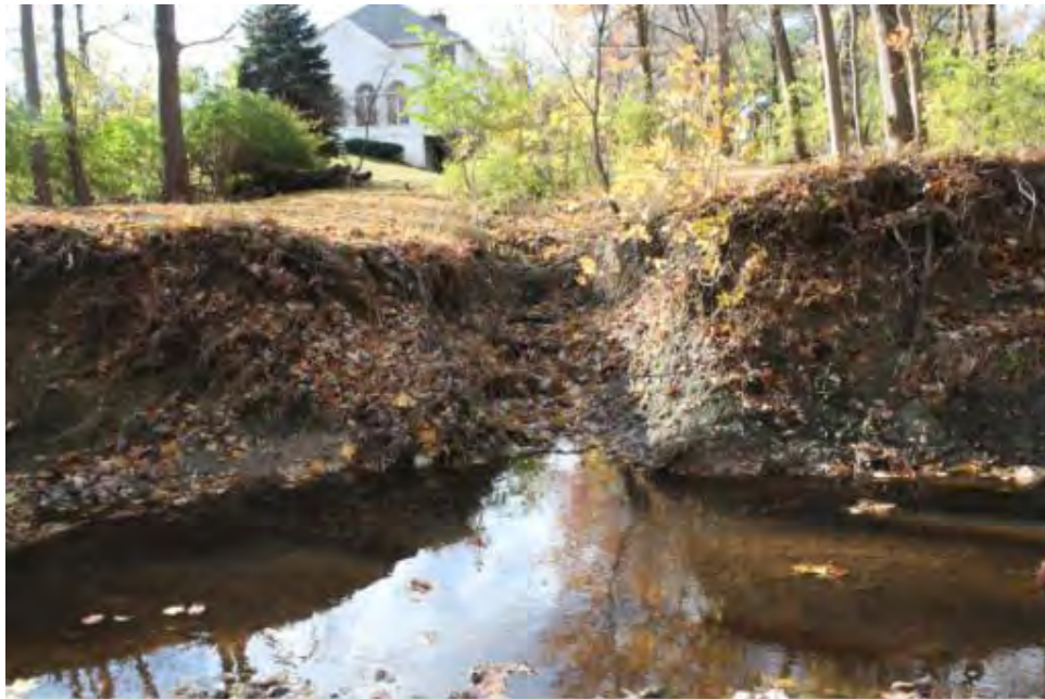
Figure 2: Severly eroded banks at a confluence
