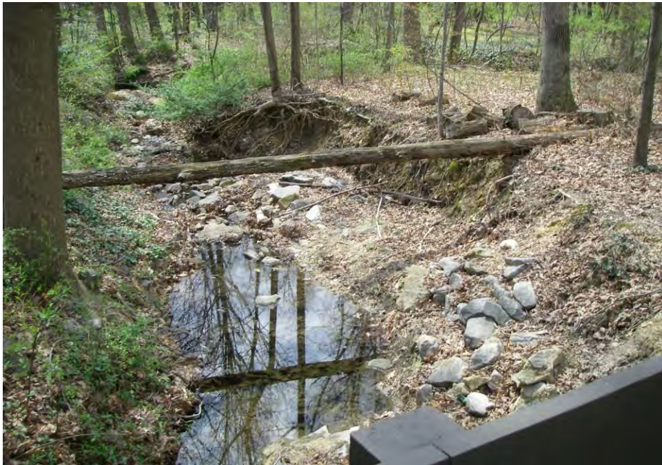
Site Photo: Moderate bank erosion
