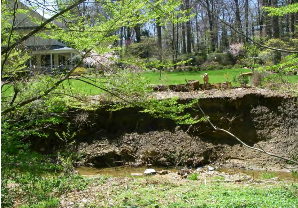
Site Photo: Severe erosion next to sanitary sewer and property owner
