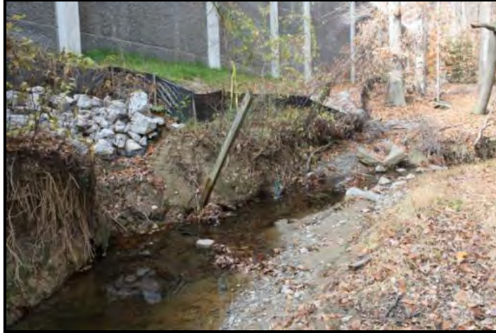
Figure 1: Severe bank erosion just upstream of I-495
