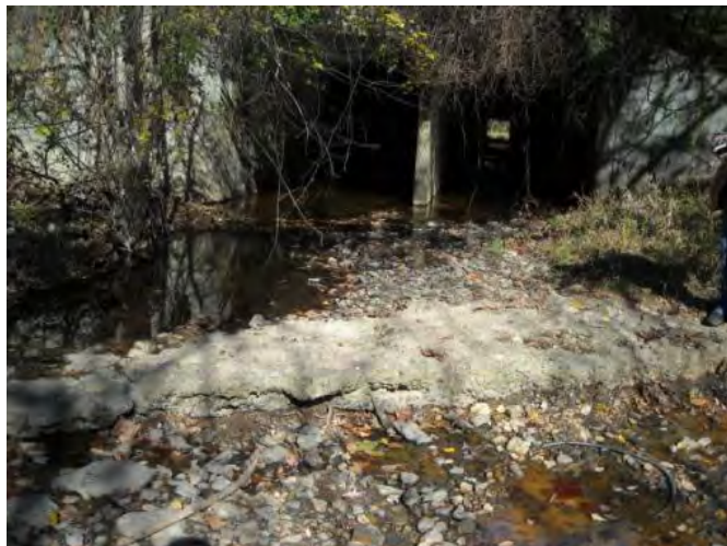
Figure 3: Existing concrete utility casing within the channel near the culvert under I-66
