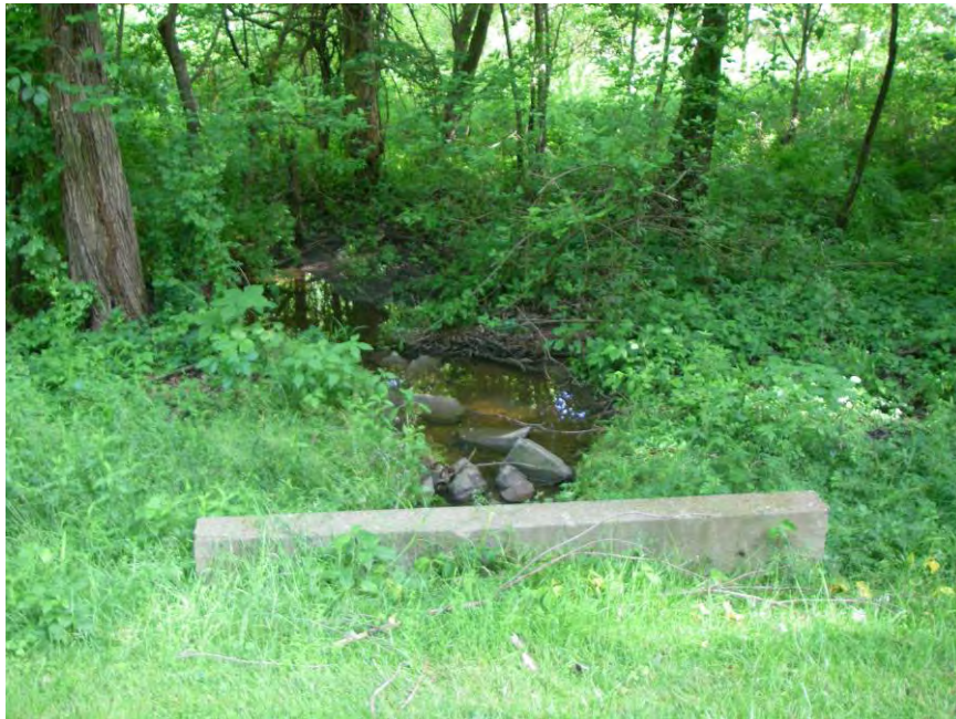
Site Photo: Inflow into Facility
