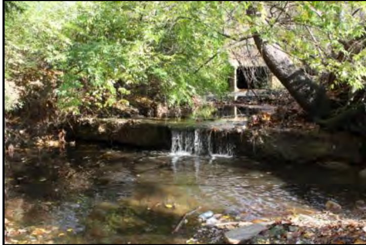
Figure 1: Severe headcut just downstream of the culvert under CottageStreet
