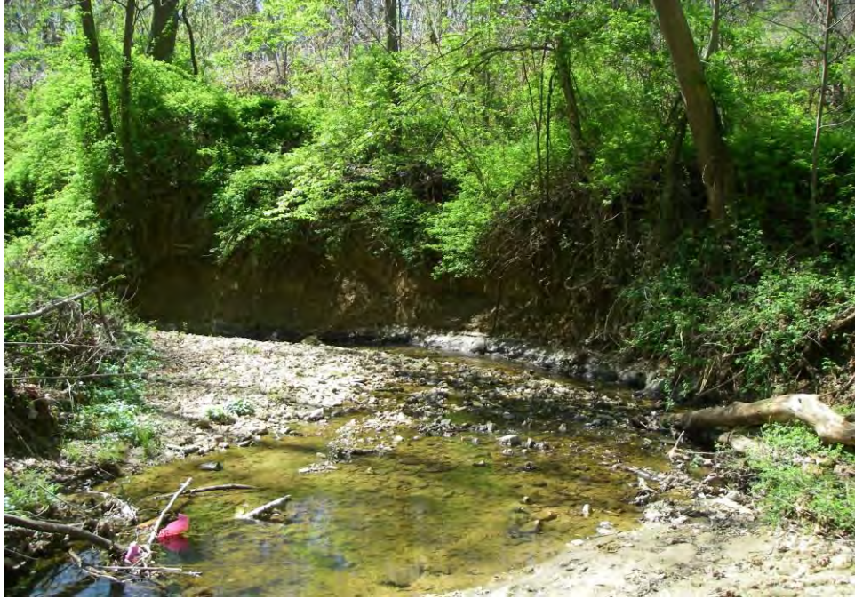
Site Photo: Severe erosion on meander bend upstream of Little River Turnpike
