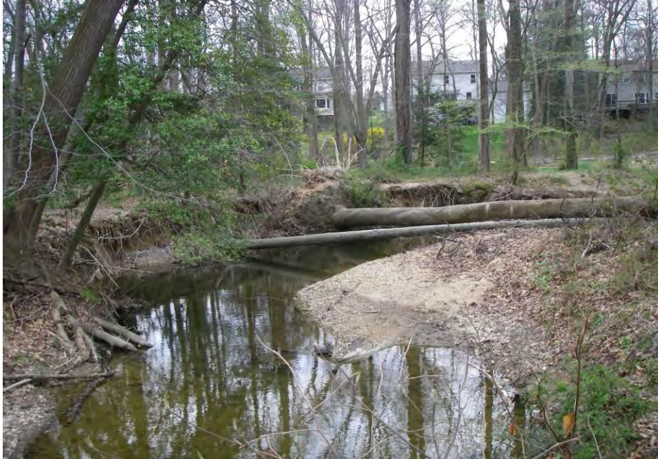
Site Photo: Severe meander bend erosion
