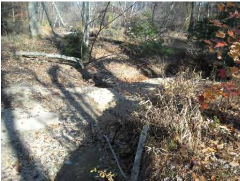
Figure 2: Overflow channel with large sand deposits
