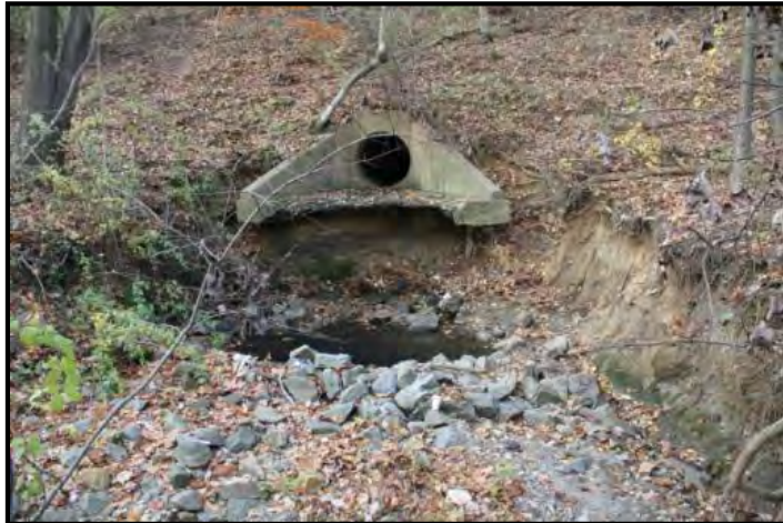
Figure 2: Severe erosion and downcutting at a storm drain outfall
