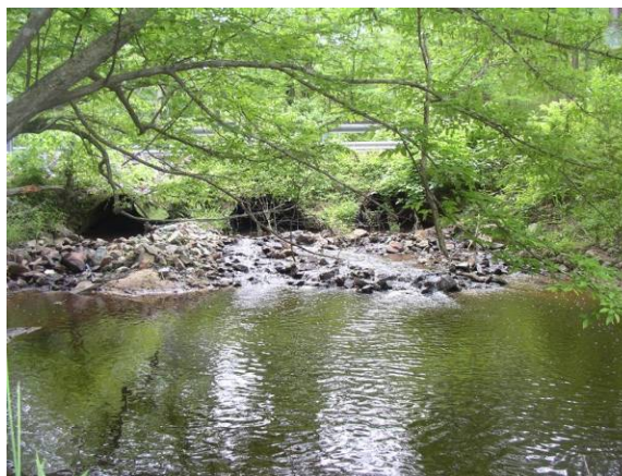
Figure 4-15: Obsolete culvert (Source: KCI)
