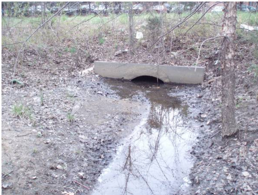
Site photo: Sediment-filled channel and discharge point to Long Branch South
