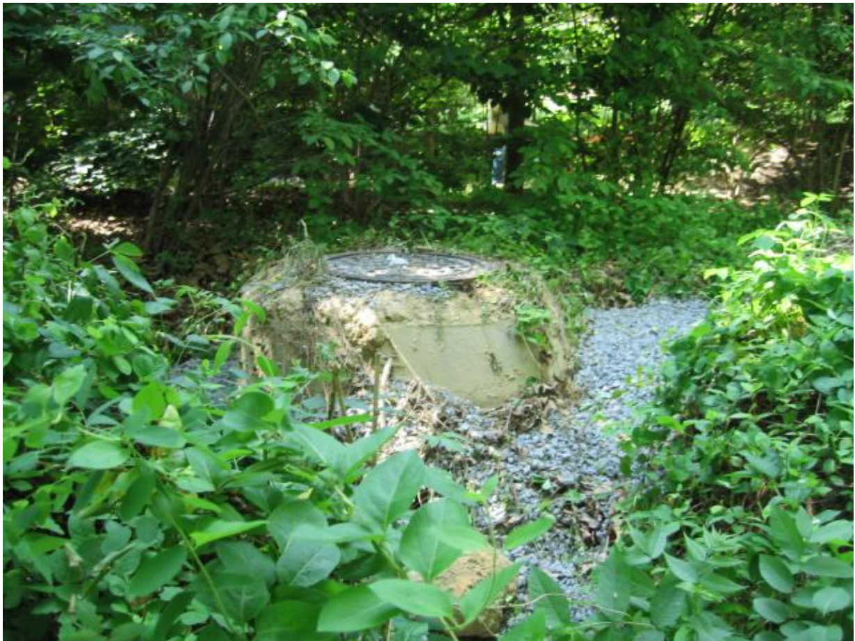
Fig. 5: Example of severe erosion at the rain garden's embankment (RG-10)
