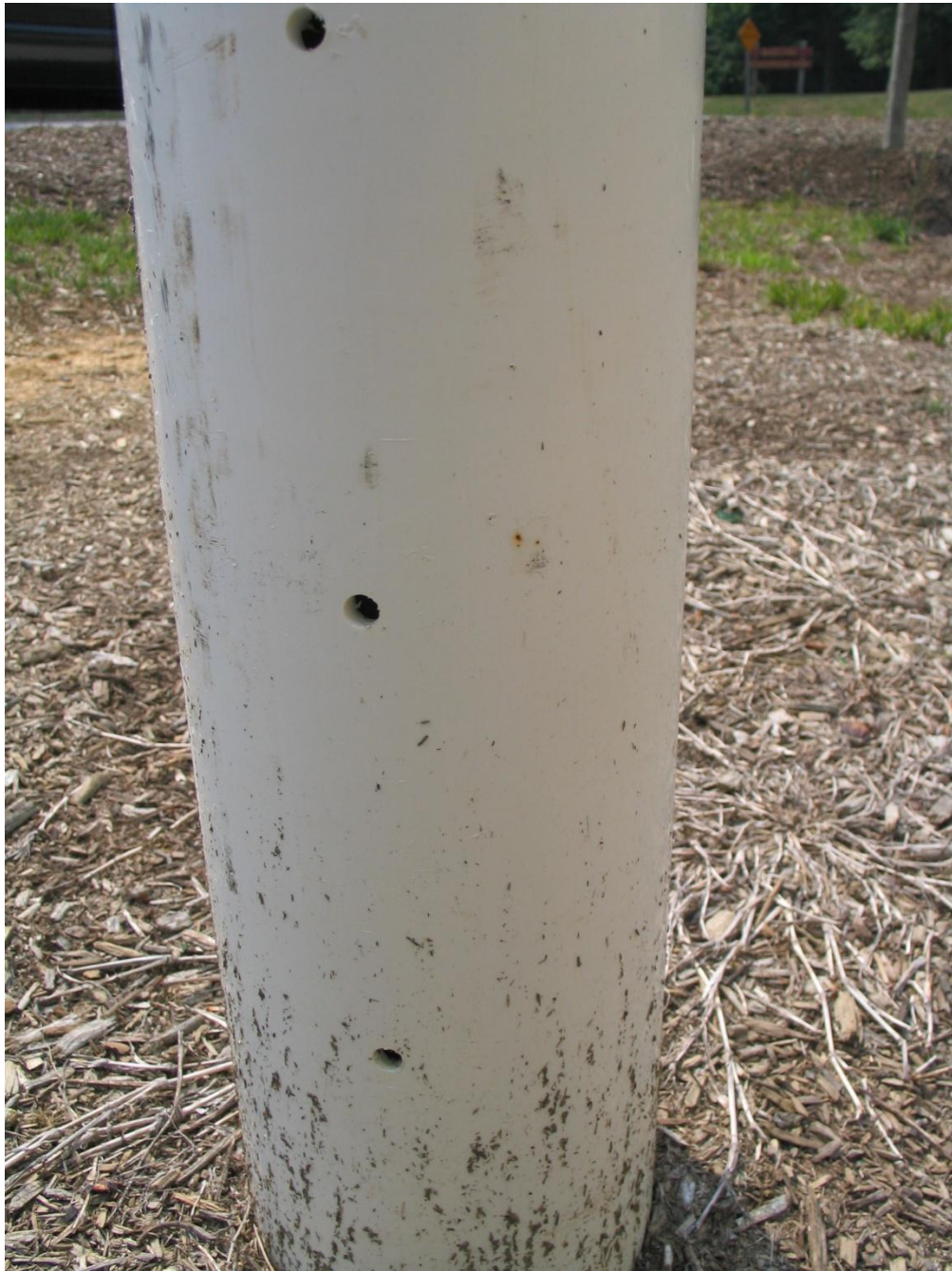
Fig. 4: Example of a perforated observation well (cleaning well) in one of the surveyed rain gardens (RG-11)
