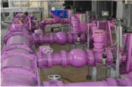
Fairfax County Water Reuse Facilities
