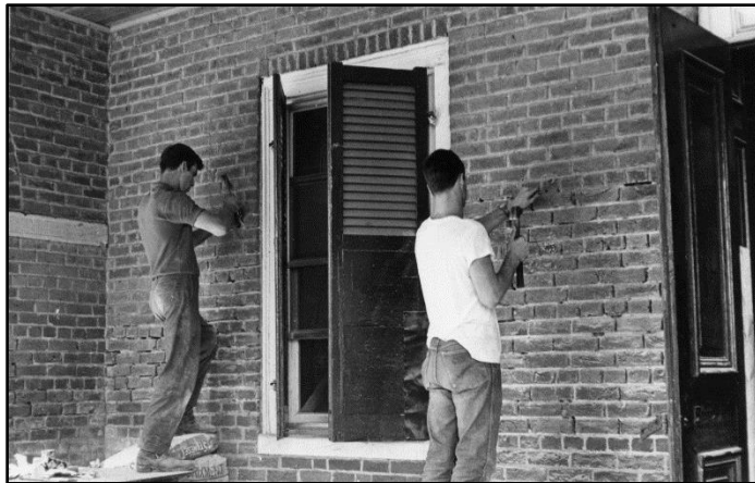
Repointing Bricks in the Historic Courthouse Arcade, 1967, Courtesy of Fairfax City Museum
