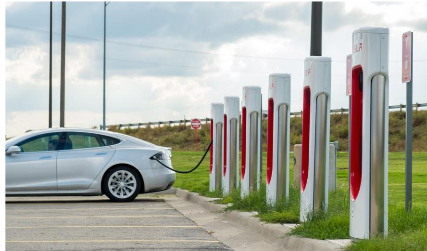
Electric Vehicle Charging
