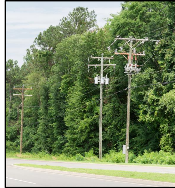
Distribution Line: Overhead Structures
