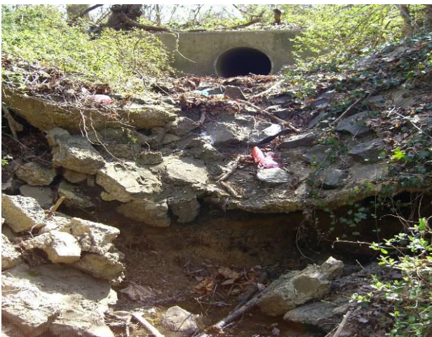
Figure 4-9: An eroded outfall
