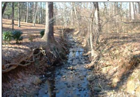
Eroded stream banks at a tributary to Dead Run near Churchill Road
