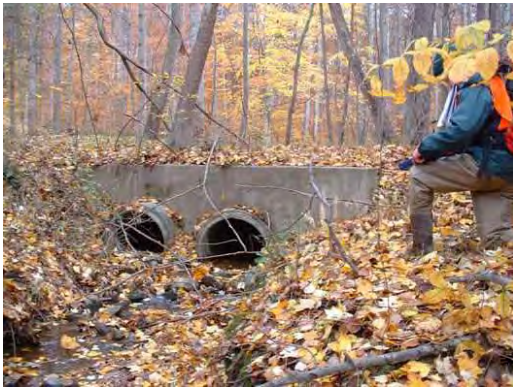
Photo 3.13 A double barrel culvert (PHPH025.C002) near Havenner Court has a minor impact on the stream
