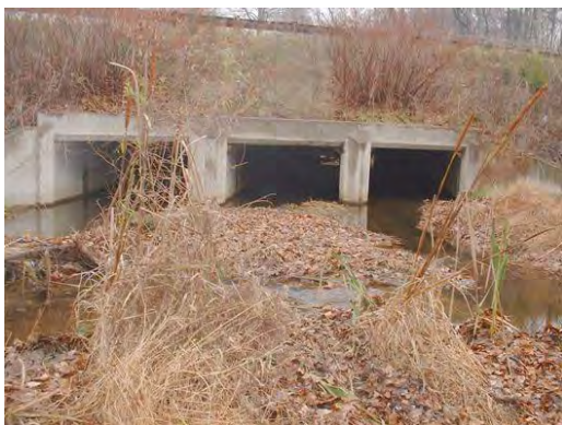
Photo 3.1 A triple box culvert (PHPH044.C001) has at Braddock Road has a severe impact on the stream
