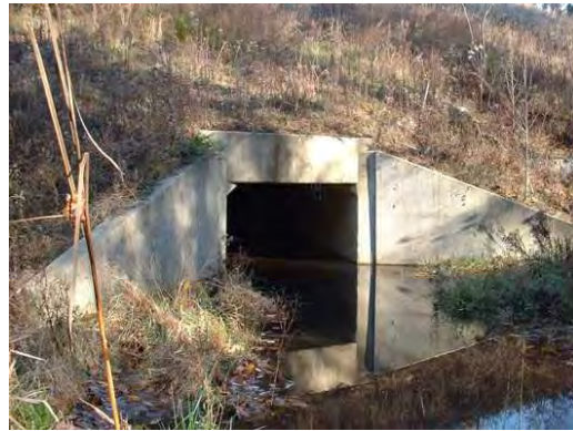
Photo 3.7 A box culvert (PHPH028.C003) near Fairfax County Parkway has a minor impact on the stream
