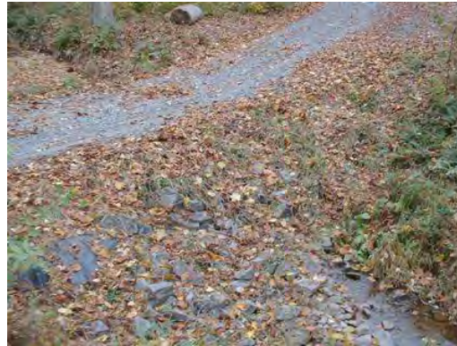
Photo 3.3 A concrete culvert (PHPI005.C002) near Quiet Brook Road has a severe impact on the stream
