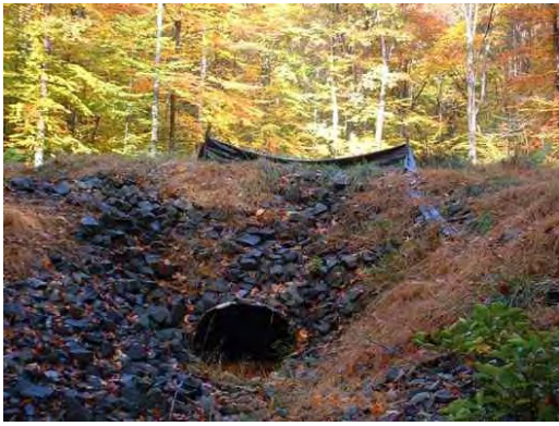
Photo 3.17 A culvert (PHPH014.C001) at Great Oak Lane has a minor impact on the stream
