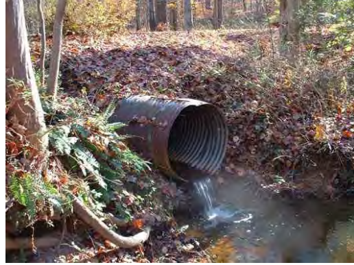
Photo 3.5 A culvert (PHPH039.C002) at McDuffie Lane has a minor impact on the stream
