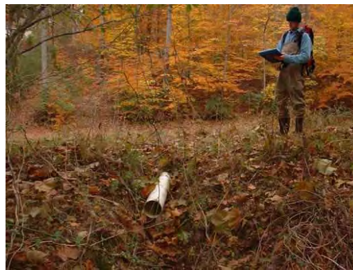
Photo 3.16 A storm drain pipe outfall is causing moderate erosion
