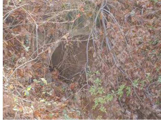
Photo 3.9 A culvert (PHCC005.C002) at Knollbrook Drive has a minor impact on the stream
