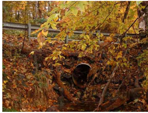
Photo 3.18 A culvert (PHPH009.C001) at Clifton Creek Drive has a minor impact on the stream
