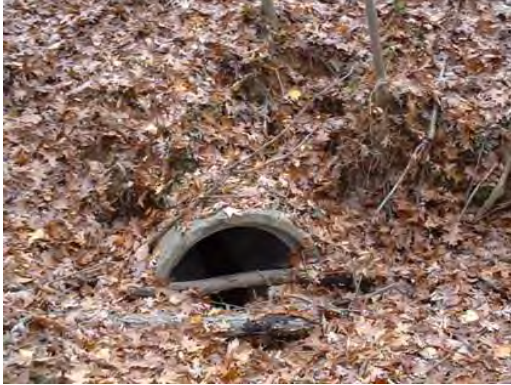
Photo 3.8 A culvert (PHCC004.C008) at Knollbrook Drive has a moderate impact on the stream
