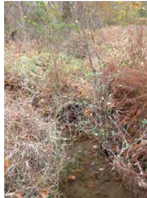
Photo 3.20 A culvert (PHPH006.C001) at Dunquin Court has a severe impact on the stream
