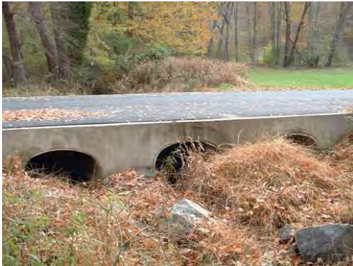
Photo 3.19 A culvert at (PHPH005.C001) Dunquin Court has a minor impact on the stream
