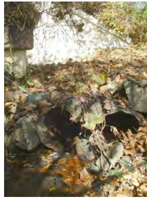
Photo 3.14 A double barrel culvert (PHPH020.C001) near Colchester Road has a minor impact on the stream
