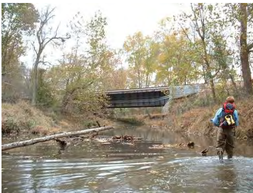
Photo 3.15 An iron bridge (PHPH014.C001) at Chapel Road has a minor impact on the stream
