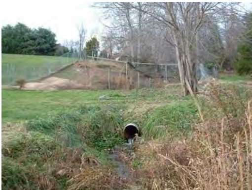
Photo 3.12 A storm drain outfall pipe near Wandering Lane has a moderate impact on the stream
