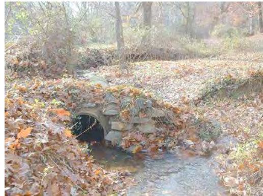
Photo 3.11 A culvert (PHCC004.C002) at Wandering Lane has a moderate impact on the stream
