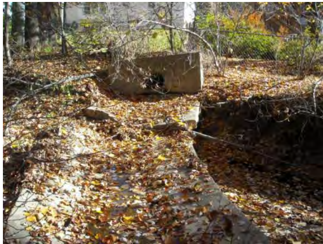
Figure 2: Eroded and undermined storm drain outfall south of Yeonas Drive
