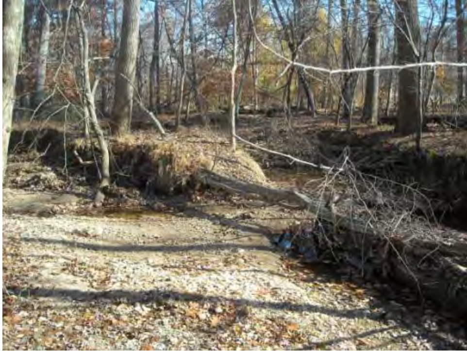
Figure 1: Overflow channel with erosion and large deposits of sand
