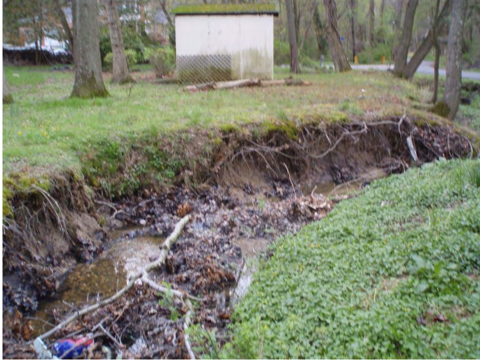
Figure 1: Eroded banks near the intersection of Pleasant Ridge Road and Walton Lane
