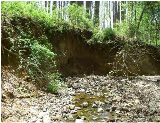
Site Photo: Severe bank erosion in channel near Collins Street
