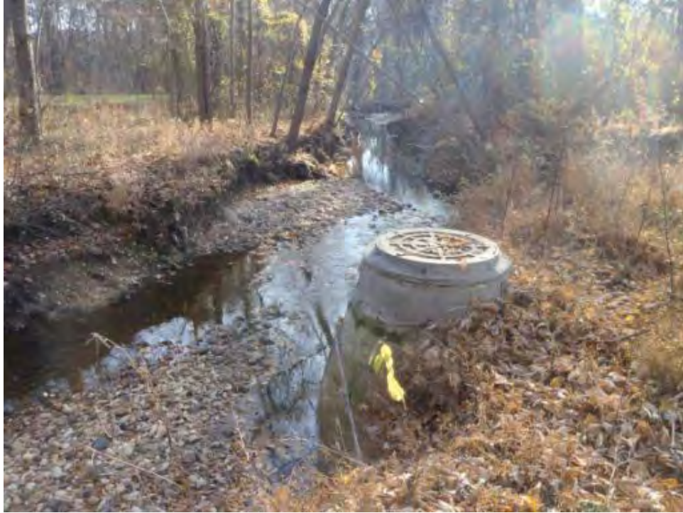
Figure 1: Exposed sanitary sewer manhole on streambank
