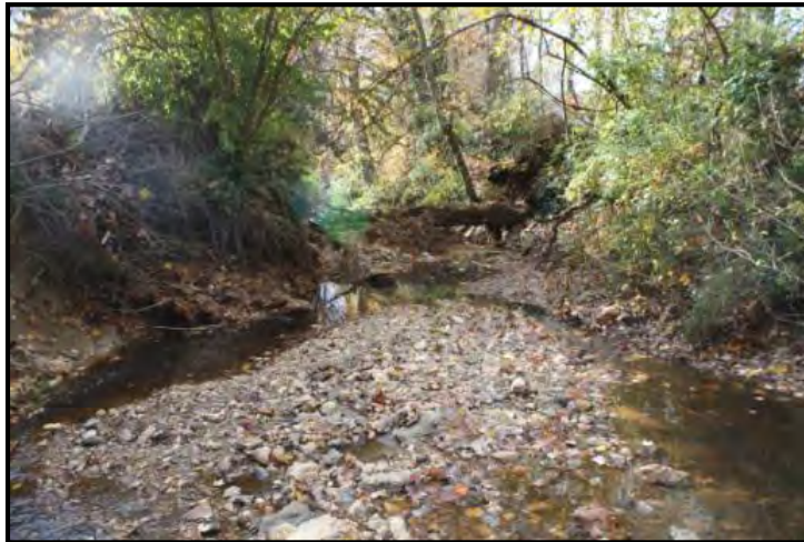
Figure 2: Severe bank erosion and channel incision
