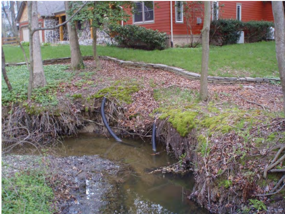
Figure 2: Channel is actively incising with eroded banks
