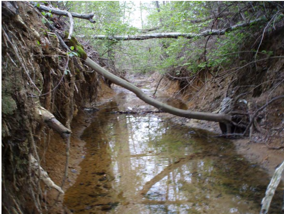
Figure 2: Incised and eroded stream channel along I-66
