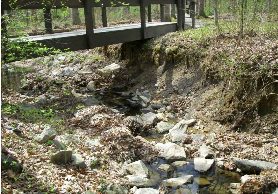
Site Photo: Moderate erosion under footbridge
