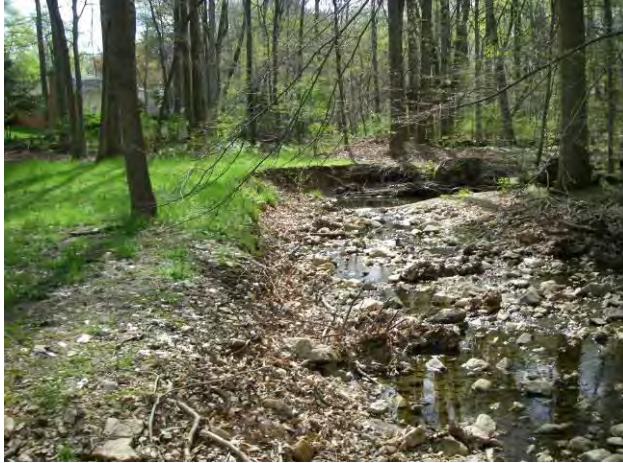
Site Photo: Upstream end with moderate erosion and adjacent sanitary sewer
