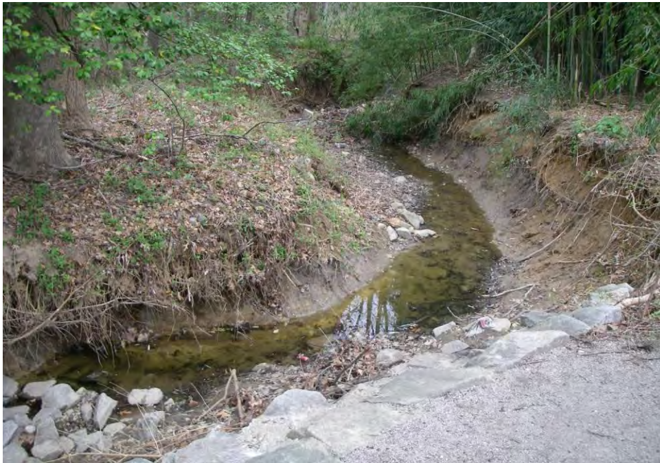
Site Photo: Erosion along tributary channel
