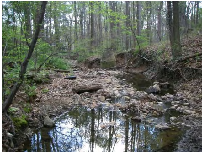
Site Photo: Sanitary sewer manhole in eroded channel
