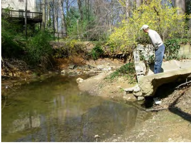
Site Photo: Downstream end with severe erosion and impacts to walking trail/storm drain inflow
