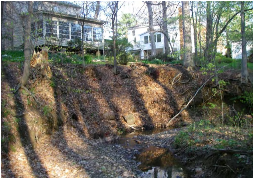
Site Photo: Erosion on meander bend adjacent to property owner
