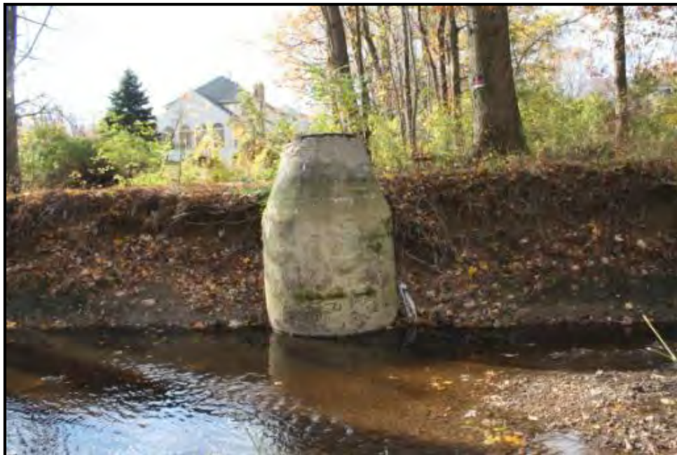
Figure 2: Exposed sanitary sewer manhole along the eroded streambank
