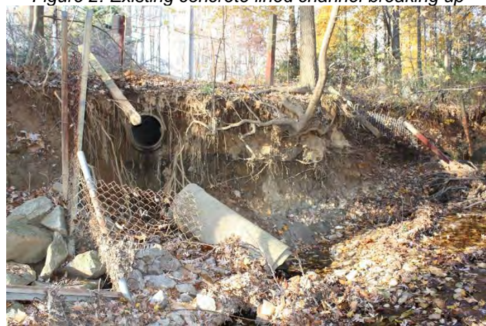
Figure 3: Severe erosion and stormdrain outfall damage
