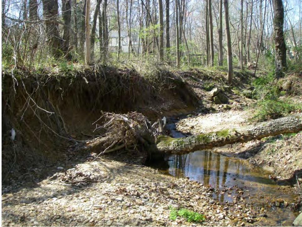
Figure 1: Eroded banks downstream of Glade Hill Drive.
