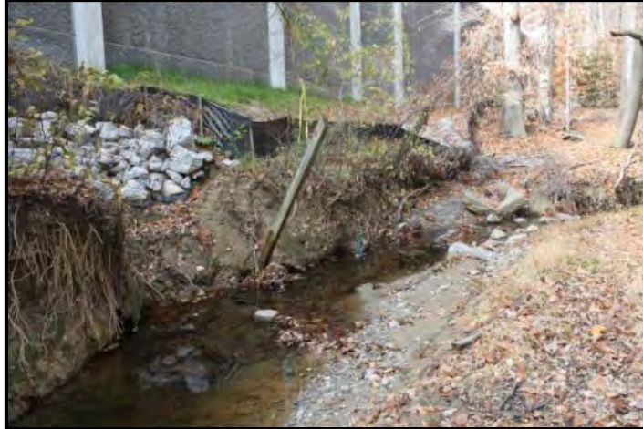
Figure 1: Severe bank erosion just upstream of I-495
