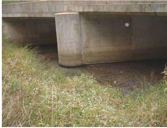
Photo 3.33 Four 10' x 15' concrete box culverts located under Collingwood Road to convey flows of the eastern tributary
