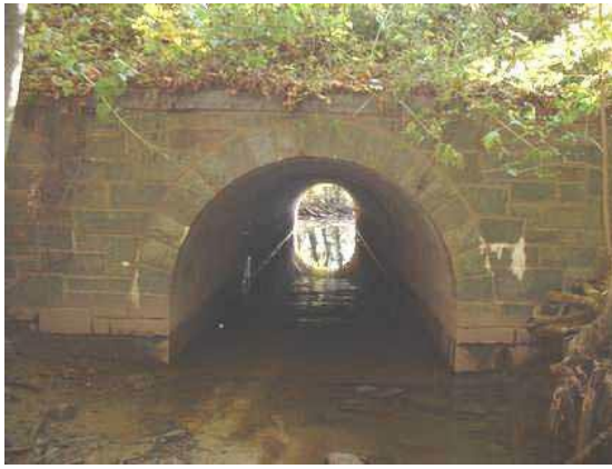
Photo 3.41 Concrete arch culvert of size 7' by 6' located under George Washington Memorial Parkway
