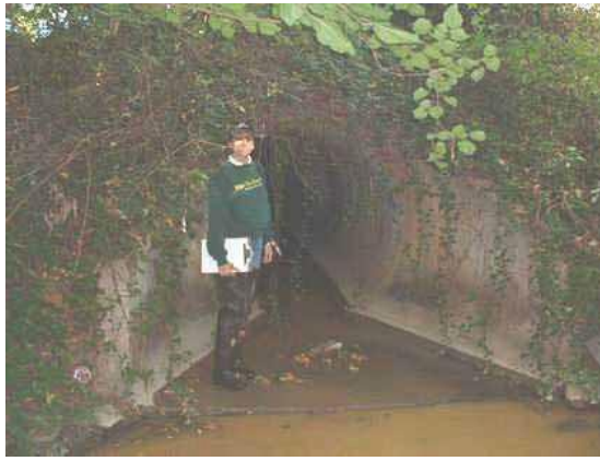
Photo 3.34 A 60" diameter concrete pipe outfall at the headwaters of the tributary to North Branch
