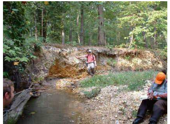
Photo 3.27 Severe erosion of 6' height observed upstream of confluence with North Branch
