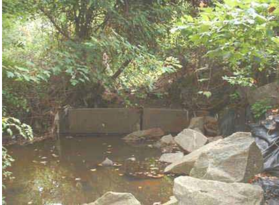
Photo 3.23 Concrete blocks obstructing the flow south of the intersection of Rollins Drive and Radcliff Drive
