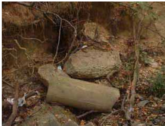
Photo 3.19 Severe erosion caused by discharge from an 18" pipe outfall west of the Mary Baldwin Drive crossing
