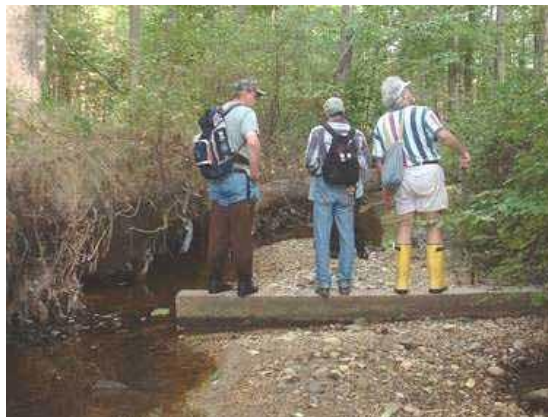
Photo 3.21 Minor erosion of the right bank at the ditch outfall north of the intersection of Paul Spring Road and Pickwick Lane
