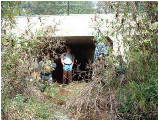
Photo 3.32 Five 12' x 8' concrete box culverts located under Collingwood Road to convey North Branch main stem flows
