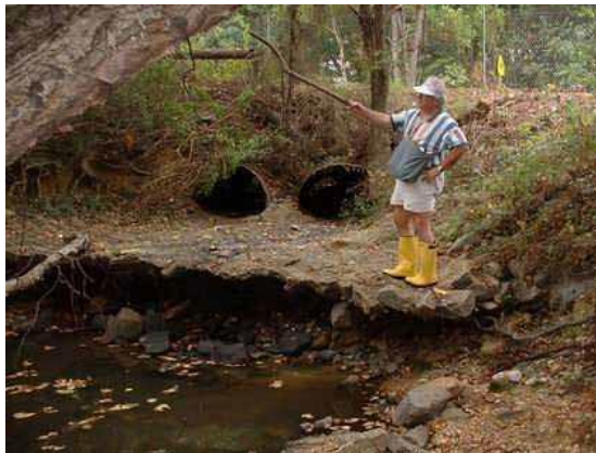
Photo 3.16 Severe erosion downstream of the Mary Baldwin Drive crossing
