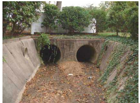
Photo 3.13 Double 3' (diameter) concrete pipes located west of Vernon View Drive
