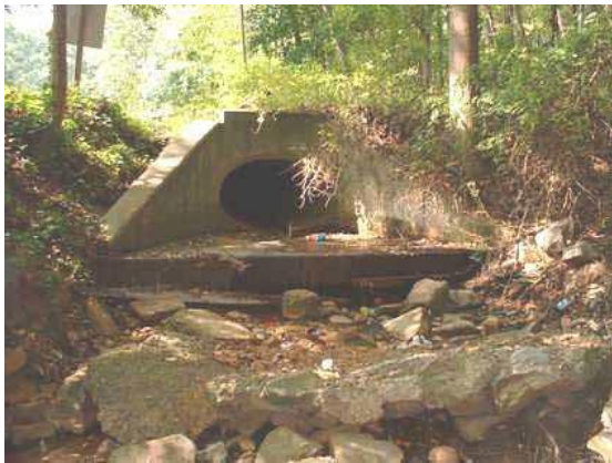
Photo 3.18 Discharge from 53"x 34" elliptical pipe outfall north of Devonshire Road caused moderate erosion on the downstream side
