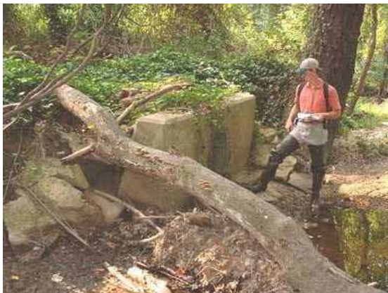
Photo 3.20 Severe erosion caused by discharge from 24" pipe outfall located north of Wellington Road
