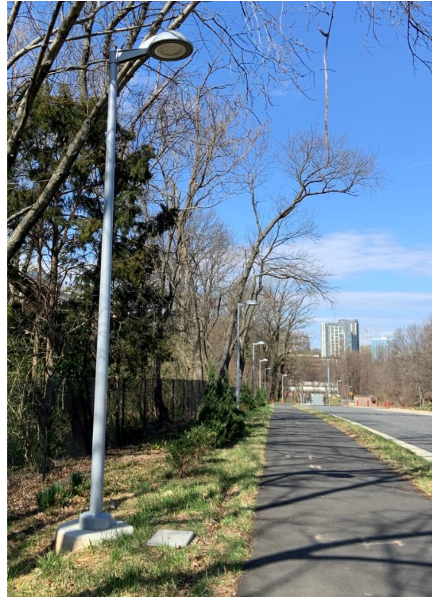
SHARED USE PATH LIGHTING
