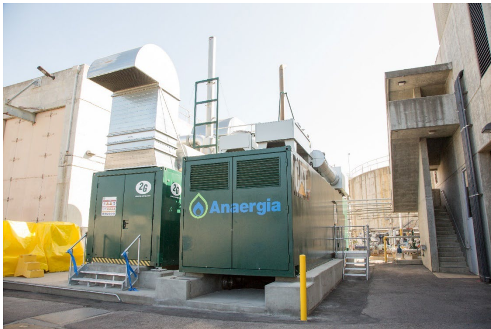
CHP Engines at Escondido Bioenergy Facility
