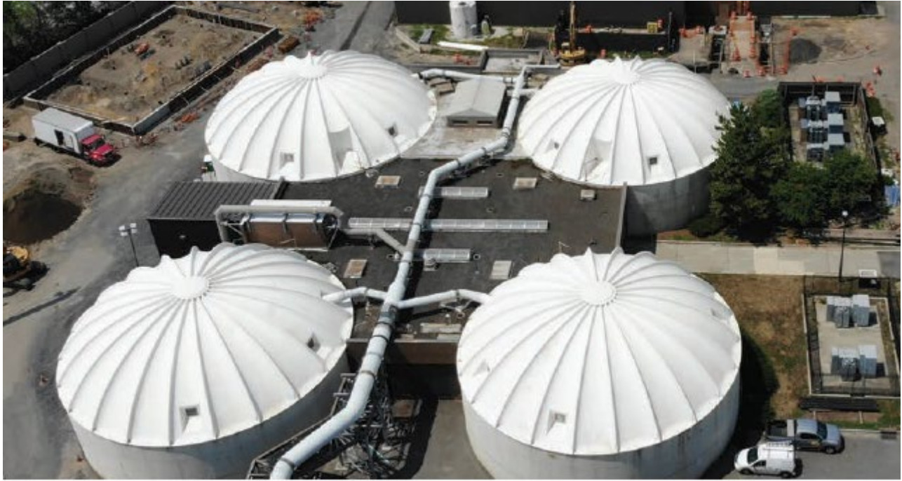
Anaerobic Digesters at Camden Bioenergy
