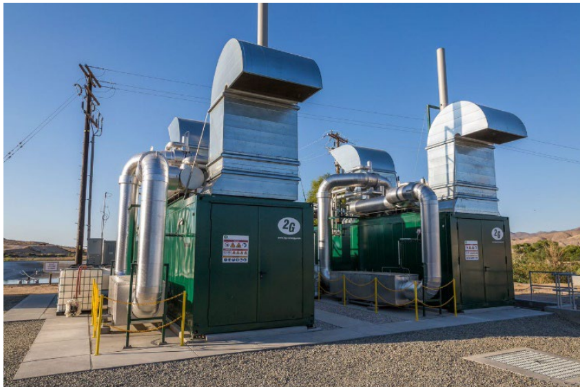
CHP Engines at VWVRA
