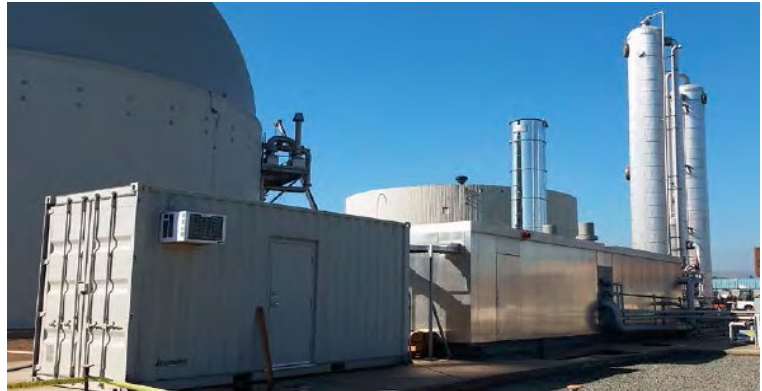
Figure 9: Biomethane Upgrading System
