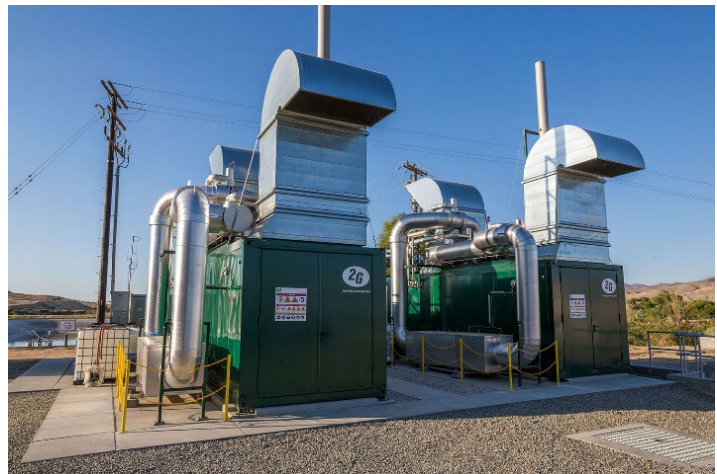
Figure 10: Anaergia's 1.6 MWe Biogas CHP at the Victor Valley Wastewater Reclamation Authority in Victorville, CA
