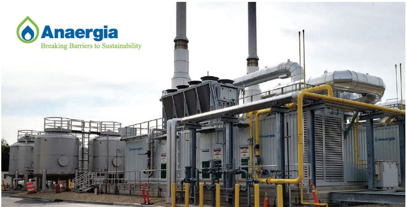
CHP Engines at Camden Bioenergy
