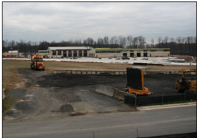
Picture of the West Ox Bus Operations Center under construction, slated for completion in fall 2008.
