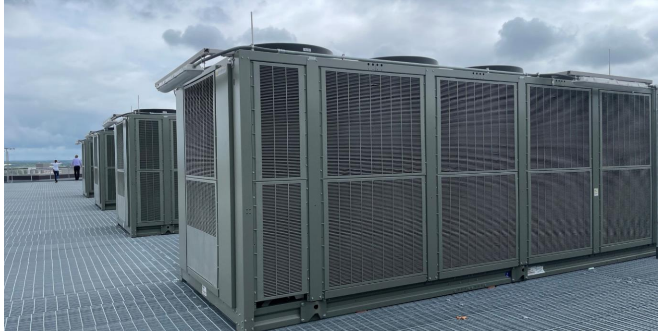
Air-cooled system, Stack Infrastructure, Manassas
