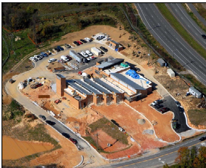
Aerial view of the construction site of the new Crosspointe Fire Station in the Springfield District.
