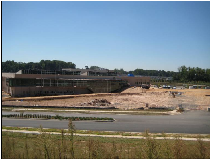
Construction is well underway on the Public Safety and Transportation Operations Center (PSTOC) facility.
