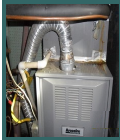
Dangerous mechanical work
