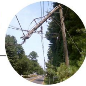
Downed utility pole in Great Falls, 2012 Derecho
