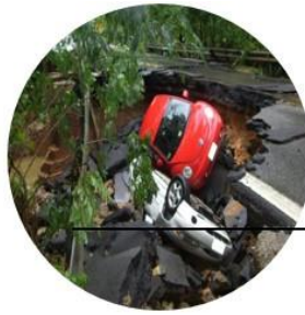
Damage along Lorton Rd., Tropical Storm Lee, 2011
