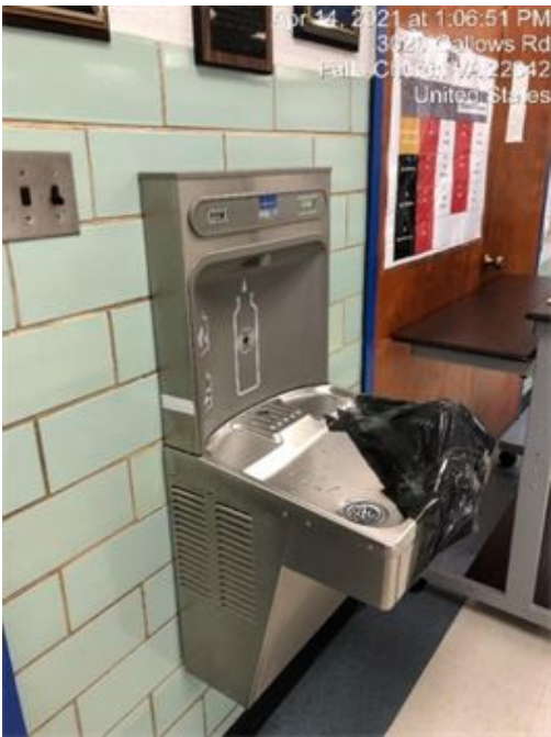
Figure 2-11. Installed Bottle Filling Station at a Current FCPS Middle School (spout currently inoperable due to COVID-19 health and safety regulations).
