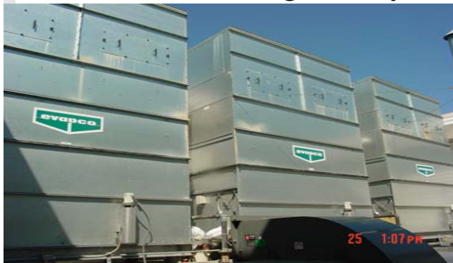
South County GC Cooling Towers
