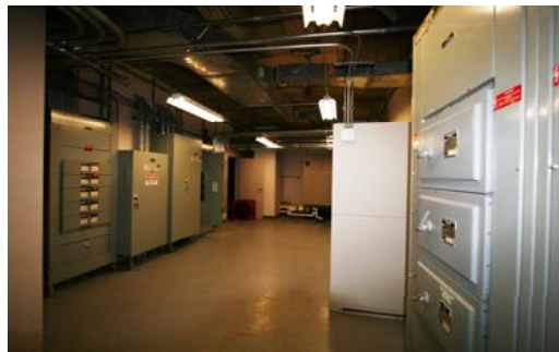
Electrical Control Room
