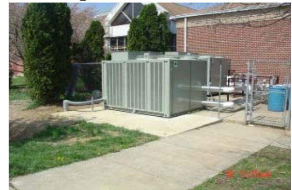
Sherwood Library Chiller
