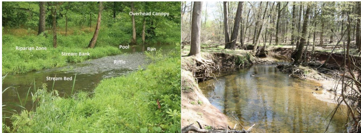
Figure 3-3: Examples of a healthy stream (left) well-connected to its floodplain, and a incised stream (right) separated from its floodplain.
