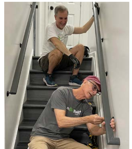
Rebuilding Together-AFF has found that installing double stair rails is an effective way to prevent falls. Photo courtesy Rebuilding Together-AFF.
