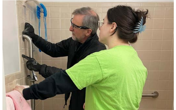
Rebuilding Together-AFF volunteers install grab bars in a shower. Photo courtesy Rebuilding Together-AFF.
