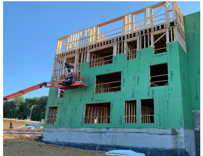
Pictured From Top to Bottom: Rendering of the Residences at North Hill Development; bldg. Retaining shotcrete stone treatment; building 2A framing.
