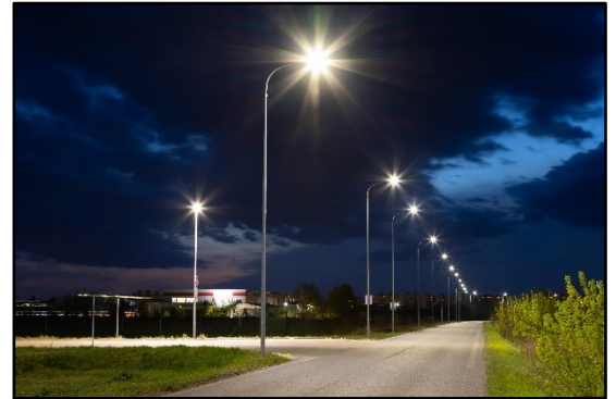
Street lights illuminating an intersection.
