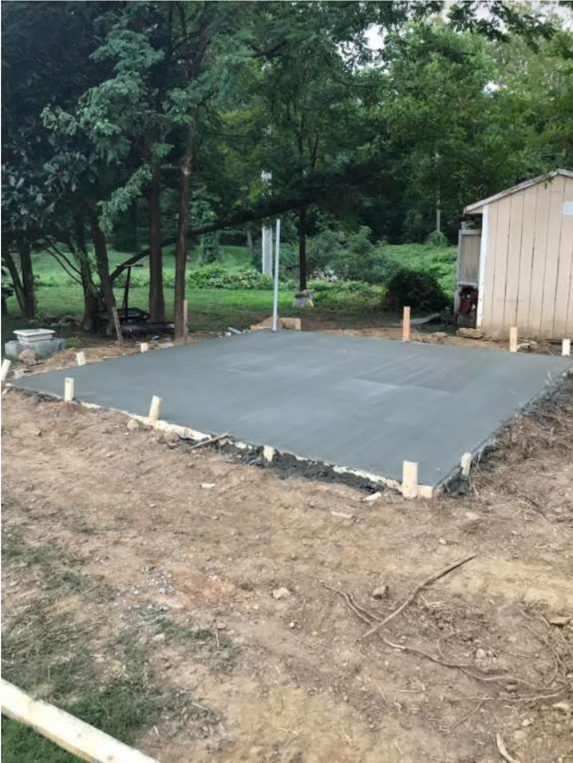
PHOTO 2: POINTING NORTHWEST, PHOTO OF SHED SLAB AND SURROUNDING AREA MOMENTS AFTER SLAB WAS FINISHED ON AUGUST 22, 2019. NOTE MINIMAL IMPACT TO TREES/VEGETATION SURROUNDING SHED SLAB.
