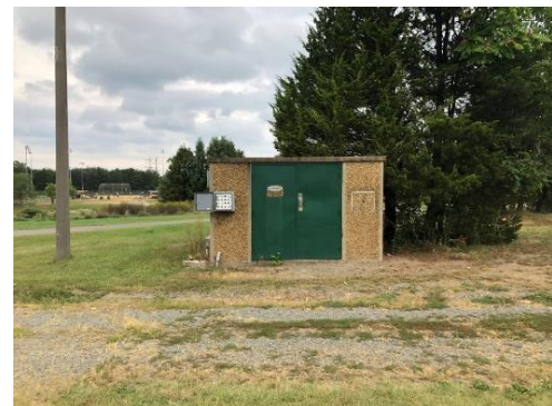
Figure 23: Electrical Control Shed
