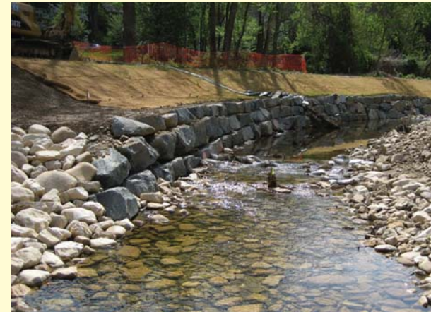
A recent stream restoration at Little Pimmit Run will improve stream water quality and stabilize the catastrophic erosion that was occurring. It cost over $500 a linear foot, but could be undermined by poor maintenance, cutting down the riparian buffer or an increase in impervious surface in the watershed.
