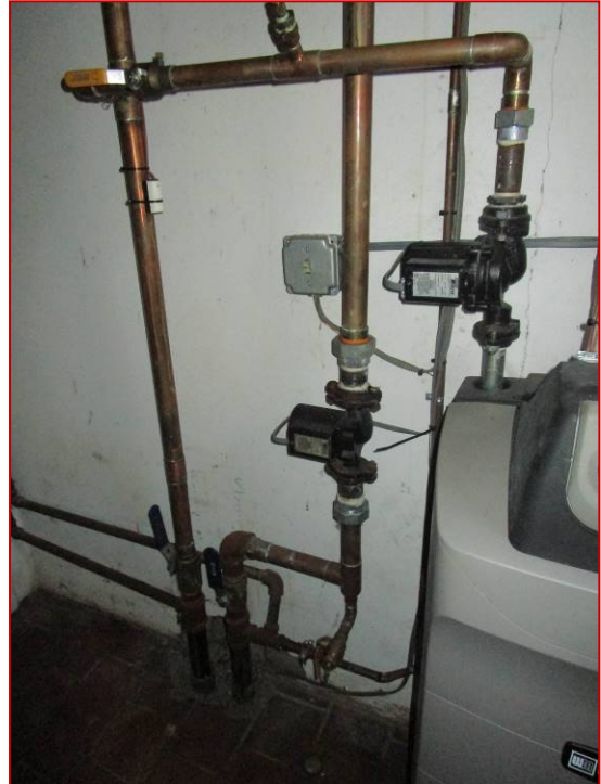
Image 10: Heating Water Piping
