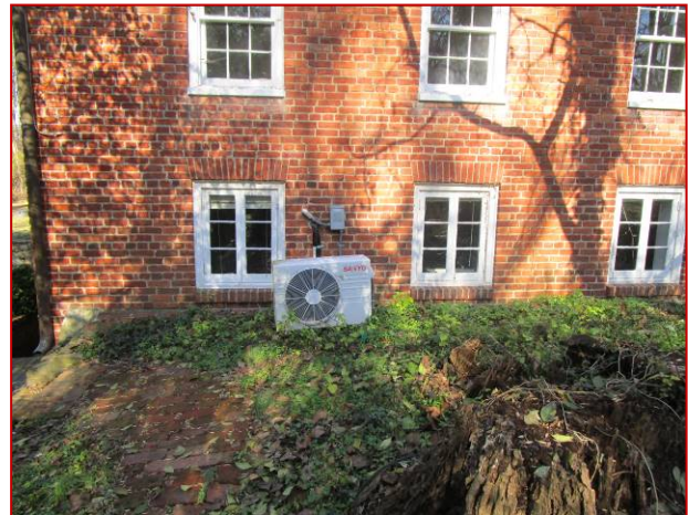
Image 2: Outdoor Condensing Unit for Kitchen
