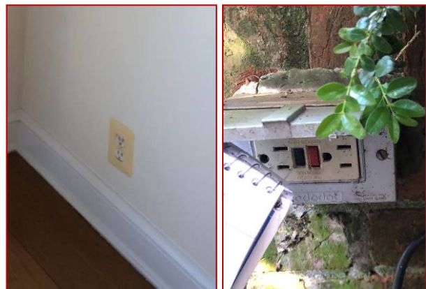
Image 30, 31: Standard Duplex Receptacle and Exterior GFCI Receptacle
