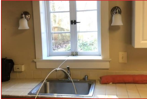
Image 32: Insufficient Number of GFCI Receptacles at Kitchen Sink
