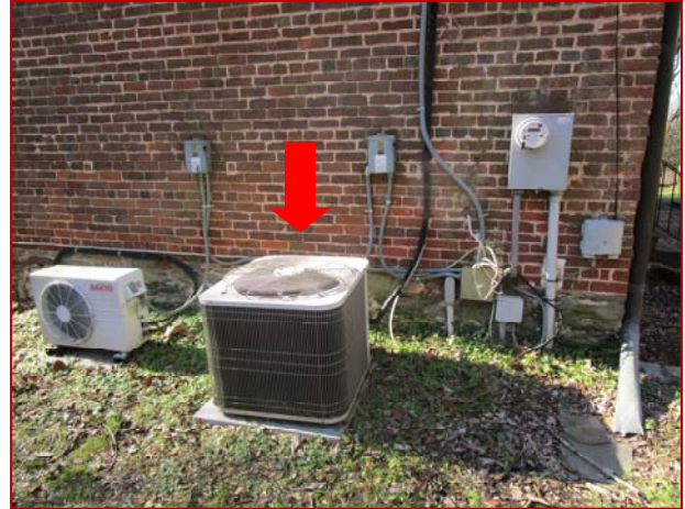
Image 6: Outdoor Condensing for Main House System
