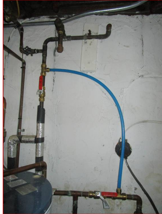
Image 15: Blue PEX Bypass Pipe
