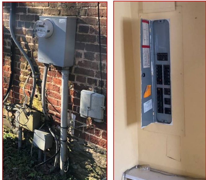
Image 27, 28: Electric Meter and 200A Main Electric Distribution Panel
