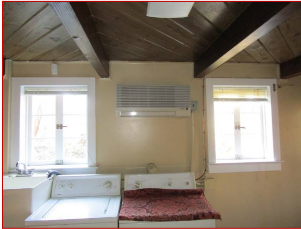
Image 1: Indoor Air-Handling Unit for Kitchen
