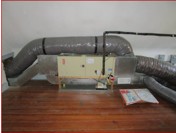
Image 5: Air-Handling Unit in East Loft
