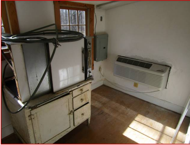
Image 13: Thru-the-Wall Heat Pump in Cottage
