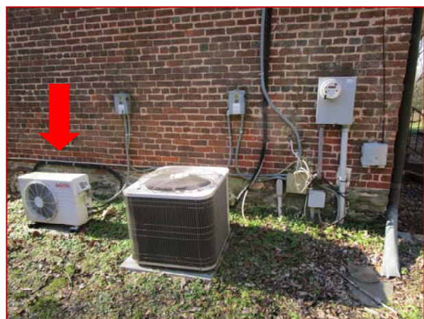
Image 4: Outdoor Condensing Unit for Cellar
