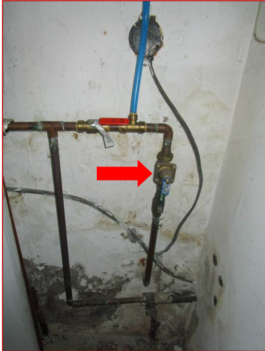
Image 14: Pressure Reducing Valve
