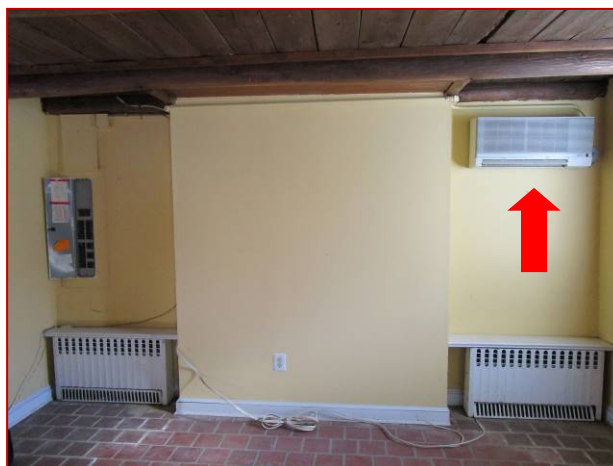
Image 3: Indoor Air-Handling Unit for Cellar
