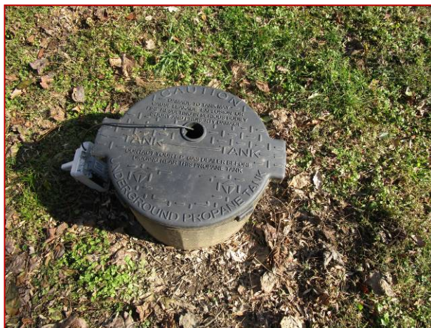
Image 11: Propane Tank Access
