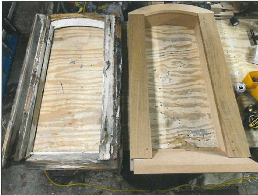
Heavily decayed window frame and its replace to match.
