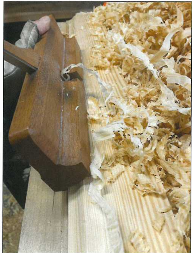
Running of moldings to match existing 18 th century examples in the Archives and in the Mansion.
