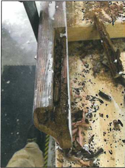
Photo showing typical decay area on a molding.
