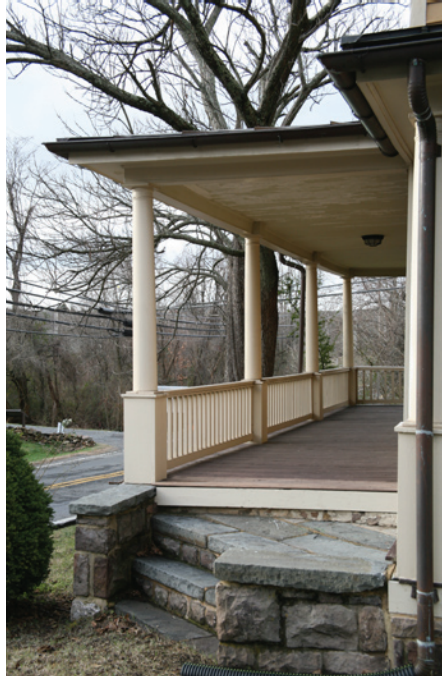
Full-width porches are found on several residences within the district, such as the Havener House example pictured here, and can provide the benefit of a shaded outdoor living space and connection with neighbors.
