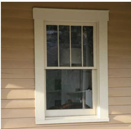
Multiple divisions in the upper sash over a single pane of glass below are seen on the Havener House.
