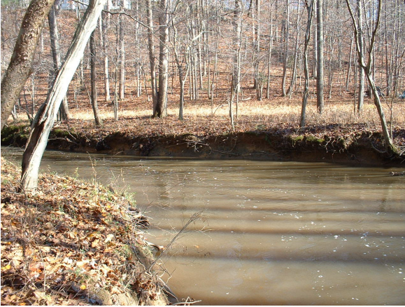
Photo 3.134 Erosion noted by field crews just east of Hunters Crest Way (DFDF009.E001).
