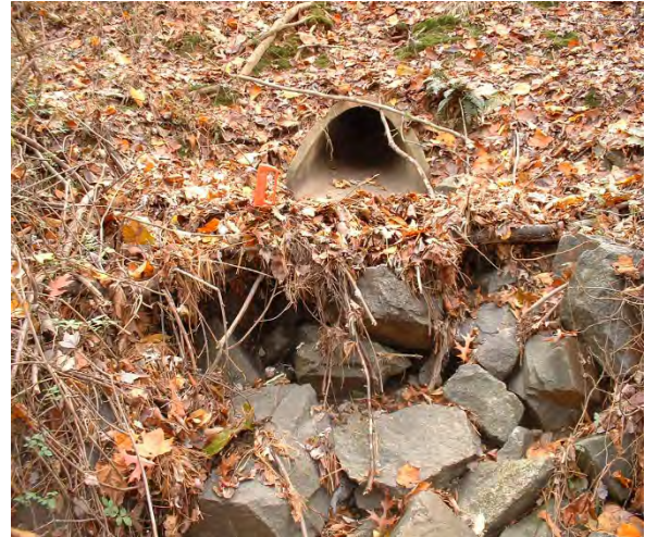
Photo 3.2 Erosion below stormwater pipe located at the end of Milburn Street (DFCH021.P001).
