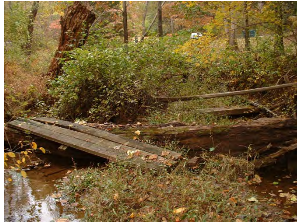
Photo 3.35 Obstruction at the northern end of Sharpers Run near the confluence with Rocky Run between the Bryan Pond and Peacock Station communities (DFSP001.T001).
