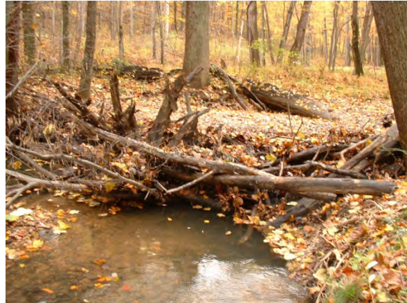
Photo 3.49 Erosion on mainstem Colvin Run downstream of Lake Fairfax before Colvin Run crosses under Hunter Mill Road (DFCR009.E001).
