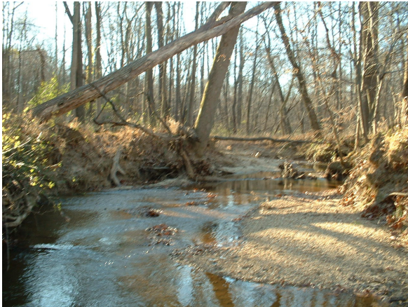
Photo 3.137 Severe erosion with moderate restoration potential located near the end of Lapham Drive (DFDF028.E001).
