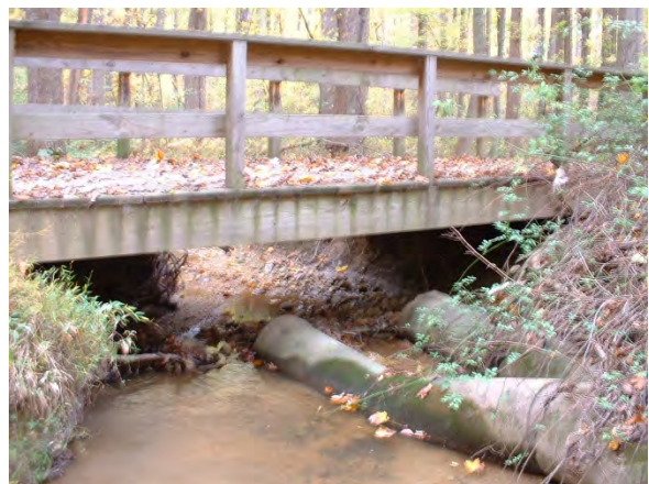
Photo 3.65 Wooden bridge where stream flow is causing moderate erosion. Located just west of Steeplechase Drive (DFGL008.C001).
