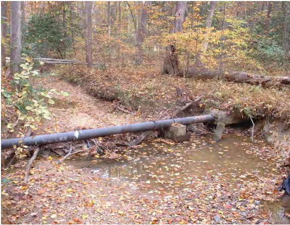
Photo 3.60 Exposed sanitary utility line crossing stream (DFSB006.U002).
