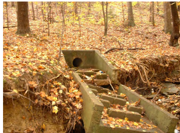
Photo 3.45 Erosion at a 12-inch outfall located just south of North Shore Drive (DFCR013.P003).
