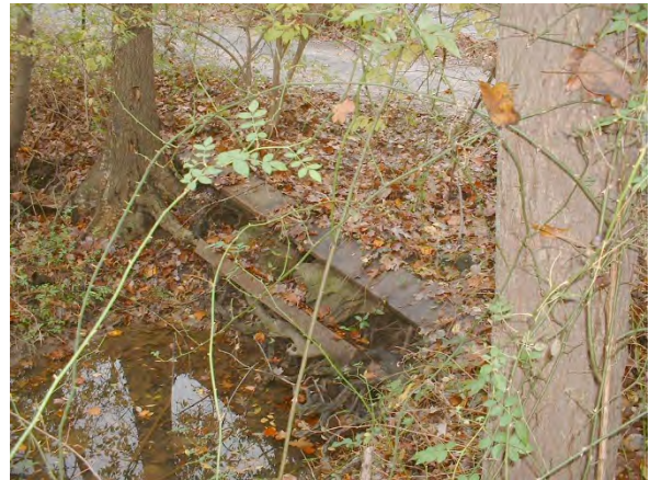
Photo 3.109 Pipe culvert at the headwaters of Angelico Branch. This is the only crossing in the watershed that has more than a moderate impact on the stream. (DFAB002.C003)
