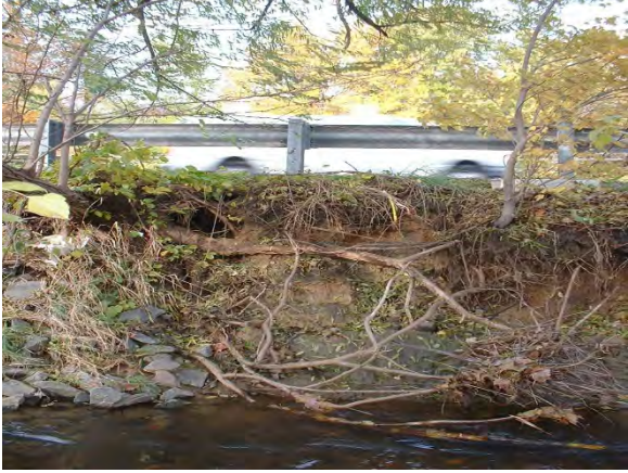
Photo 3.26 Severe erosion that could pose a threat to road safety along Route 7 to the east of Carpers Farm Way (DFCR001.E001).
