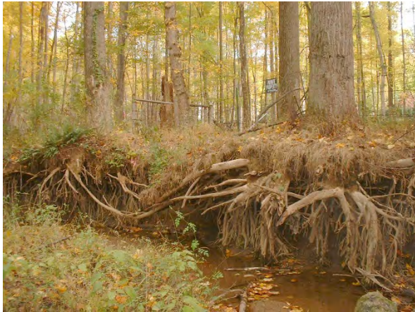
Photo 3.34 Eroding bank located east of the Lawns of Towlston Community (DFSP002.E001)
