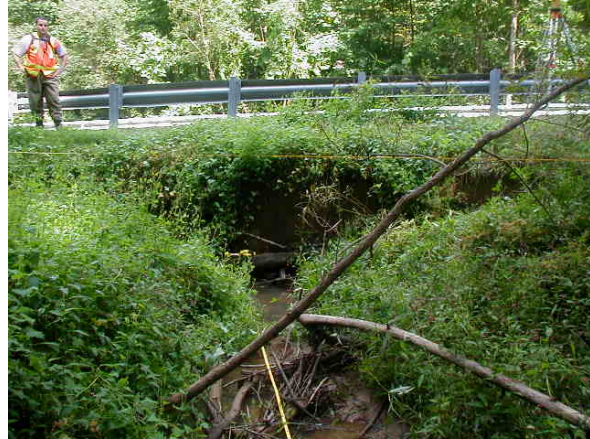
Photo 3.107 Little Difficult Run mainstem at Fox Mill Road South
