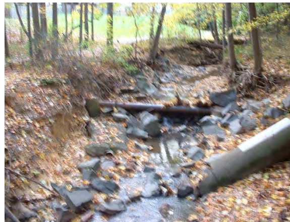
Photo 3.61 Exposed utility at the southern end of Mossy Creek Lane.
