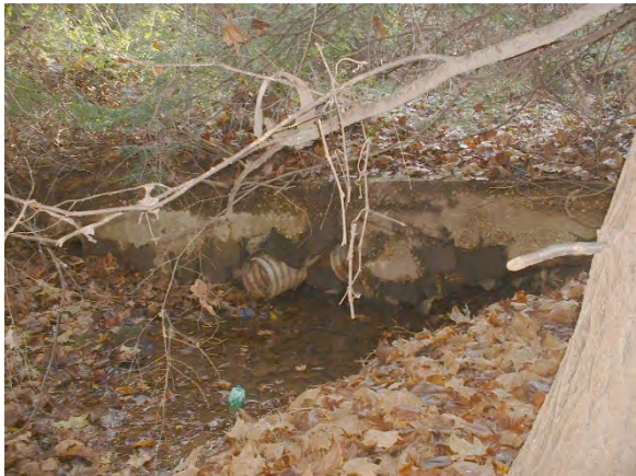
Photo 3.22 Erosion at outfall pipe located near Mill Creek Landing (DFDF003.P001).
