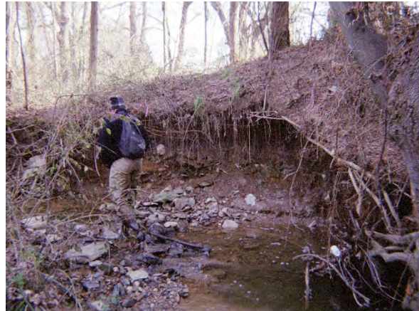
Photo 3.123 Erosion point on a tributary off of the mainstem of Rocky Branch. East of Oakton Ridge Court in the Oakton Mill Estate subdivision (DFRB010.E001)
