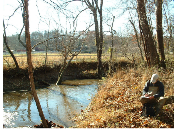
Photo 3.135 Erosion along Difficult Run located just east of Hunter Mill Road and south of the Washington and Old Dominion Railroad Trail (DFDF008.E002).
