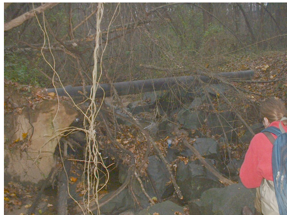
Photo 3.89 Sanitary line crossing the stream above the baseflow (DFPB010.U001).
