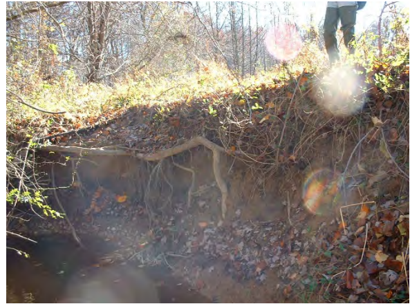
Photo 3.3 Erosion on Captain Hickory Run along Milburn Street (DFCH012.E002).
