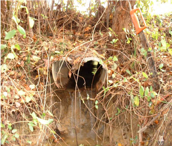
Photo 3.1 Erosion at the end of stormwater pipe located off of Collin Farm Land (DFCH021.P003).
