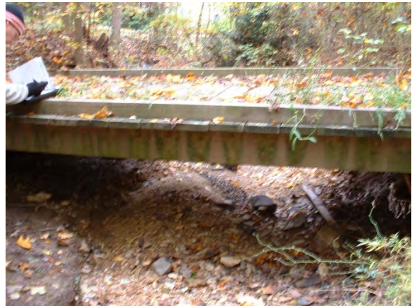
Photo 3.64 Wooden bridge where stream flow is causing moderate erosion. Located just off of Bassett Lane (DFGL008.C004).
