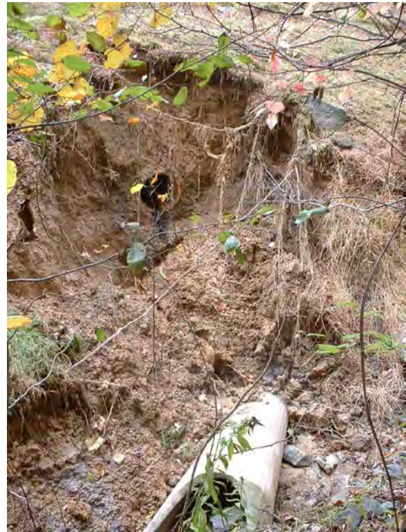
Photo 3.55 Severe erosion and pipe segment separation at a 16-inch outfall located near Alexander Bell Drive (DFSB006.P006).
