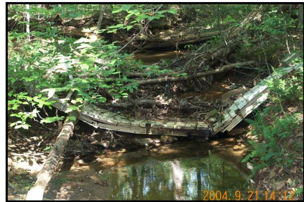
Collapsed footbridge looking upstream
