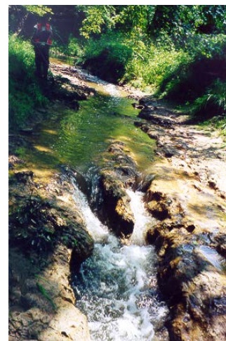
A headcut along Wolftrap Creek in the Difficult Run Watershed is indicative of erosive "downcutting."
