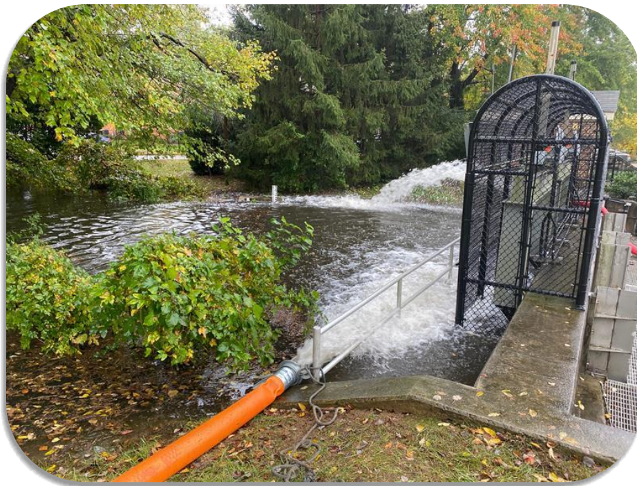
Mobile Pump deployment at the Belle Haven tidal gate during a coastal storm surge event, Fall 2021 (Fairfax County Photo)
